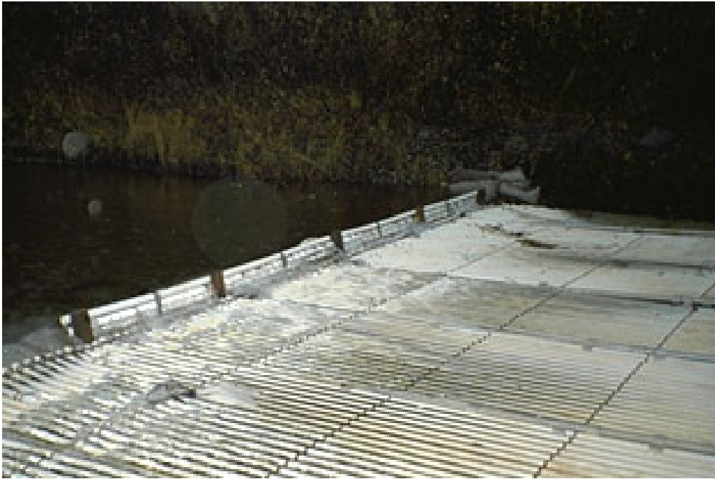
Photo Figure 3. View of low water baffle system. Note the lack of water on top of the panels.
