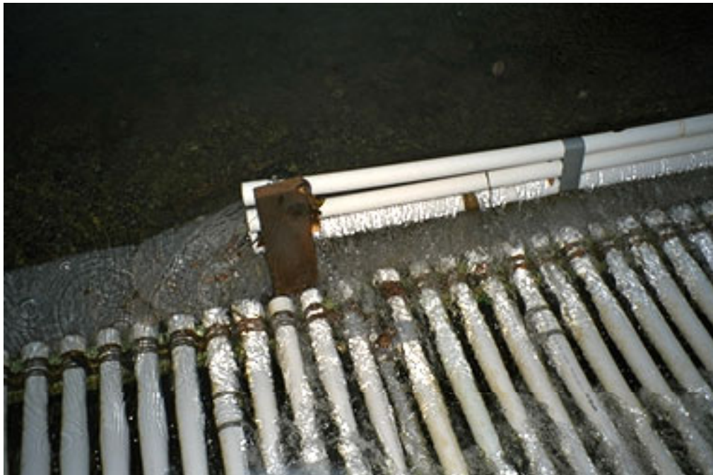
Photo Figure 4. Close-up, showing the baffle raised up off the panel. Note the 2x4 wood and the duct tape holding the P.V.C. pipes together.
