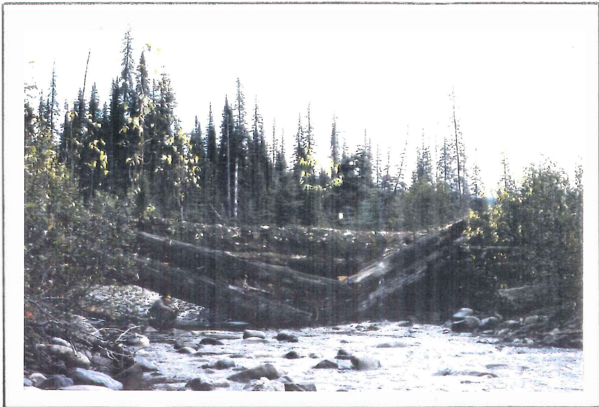
Photo 1. Bridge stringers collapsed into Natlan Creek. 93M045-Opening 9.
