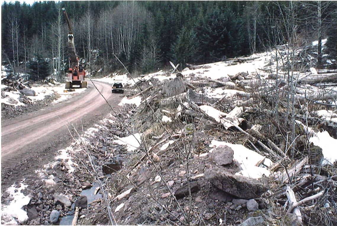
Photo 45: Alluvial fan caused by debris torrent, water flowing into ditch.
