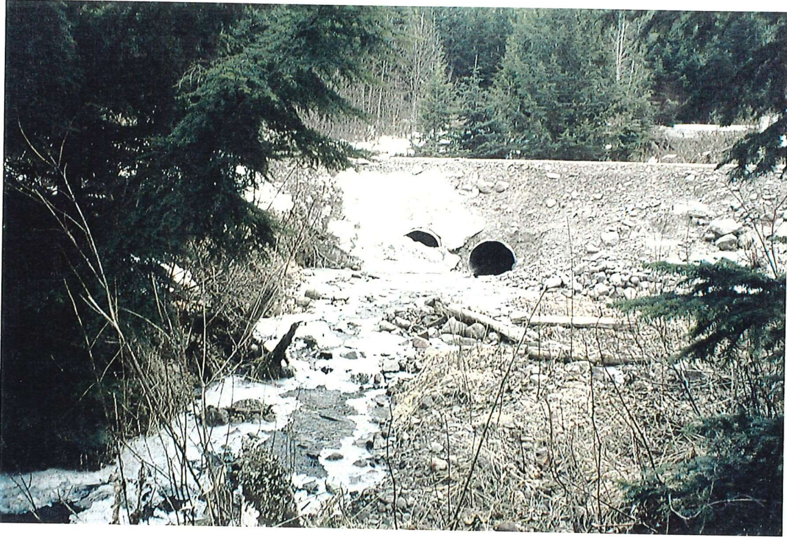
Photo 55: Degraded creek below the road.
