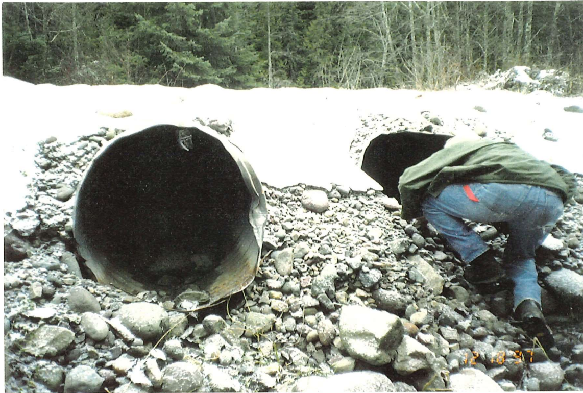
Photo 23: Perched culverts with no flow into the channel.
