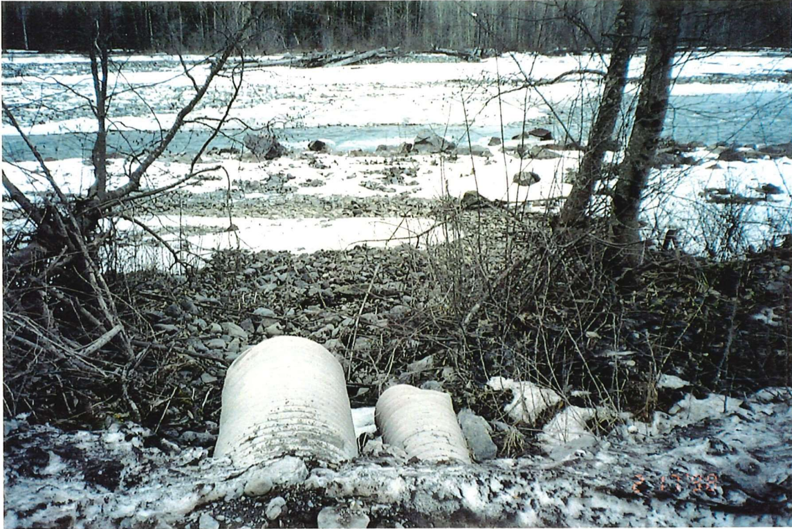
Photo 34: Water is no longer flowing from this channel (March 1998).
