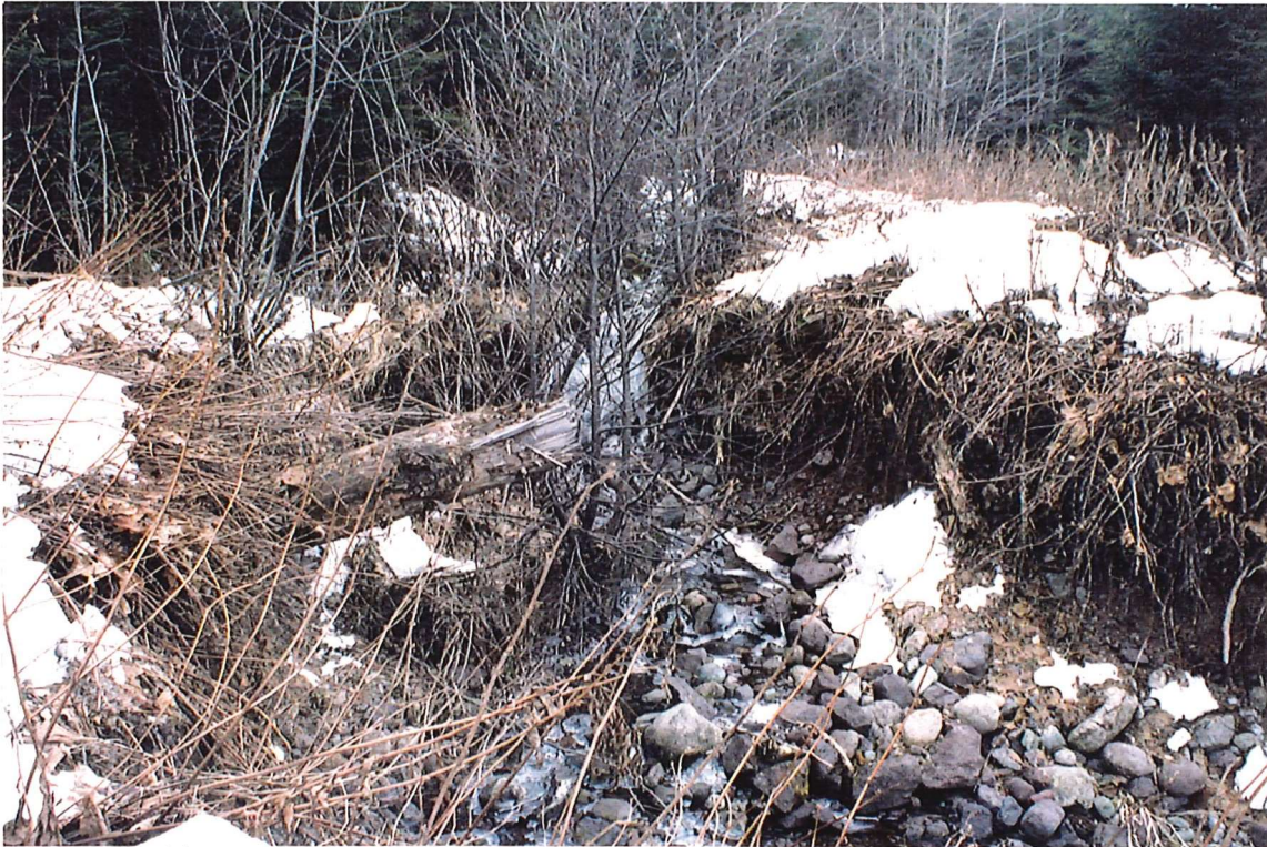
Photo 54: Above the Copper FSR, eroded bank and small water fall.
