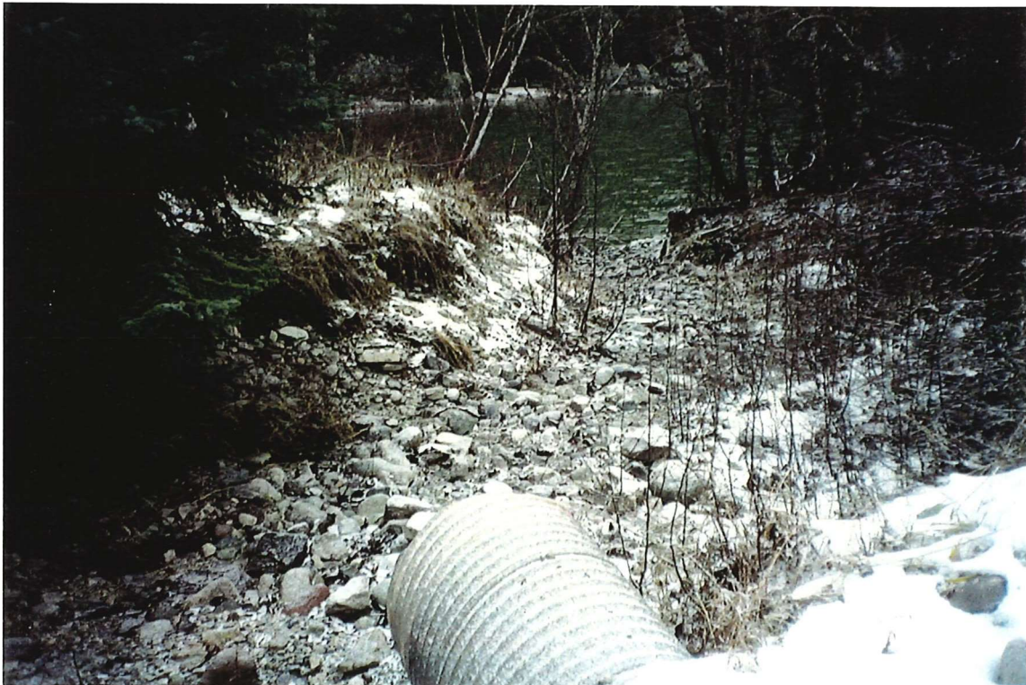
Photo 24: This culvert, just below the Copper FSR, is positioned too high.
