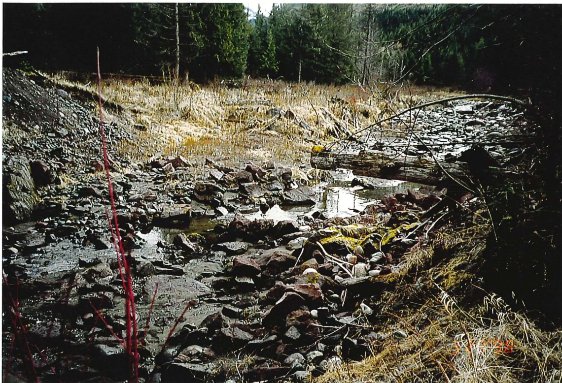
Photo 51: Looking up the channel from the washed out bridge.
