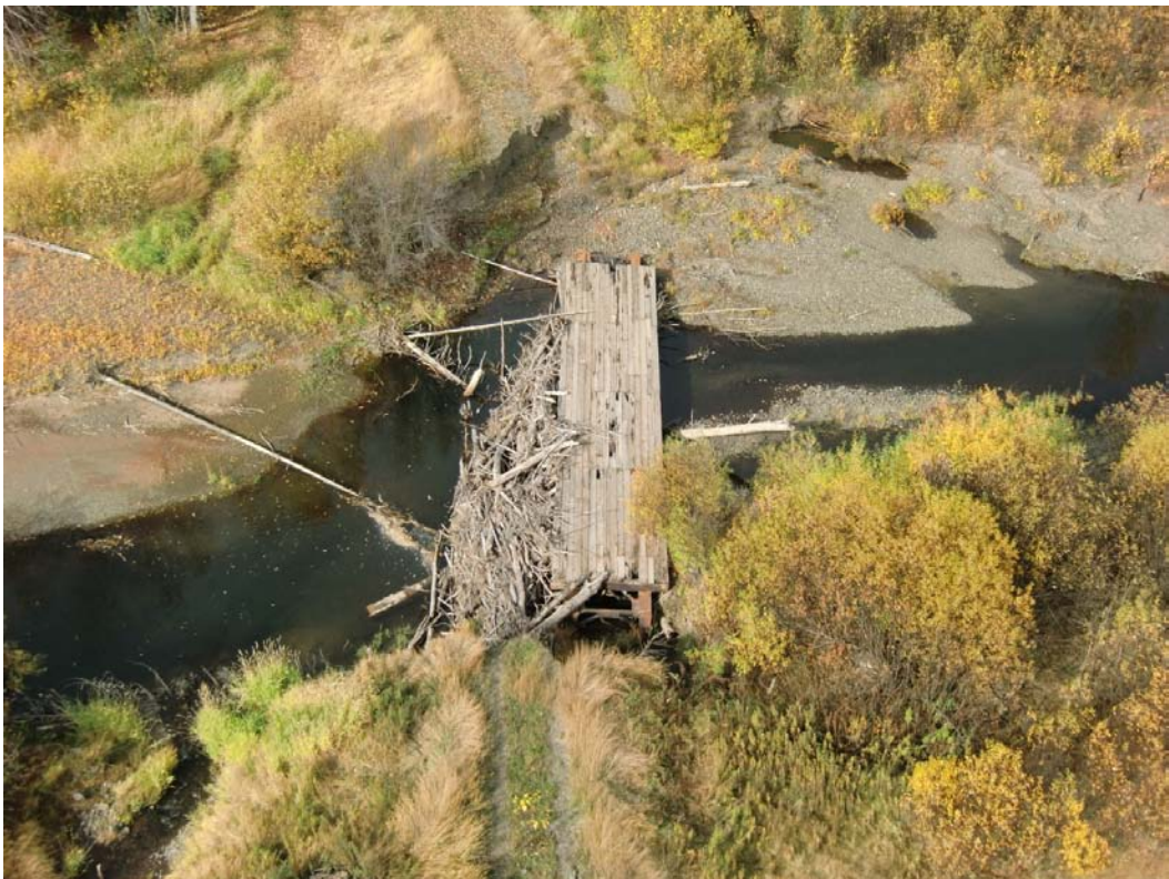
Photo 2. Strimbold bridge on Maxan Creek, debris on upstream side, known Chinook spawning on downstream side, September 29, 2015.
