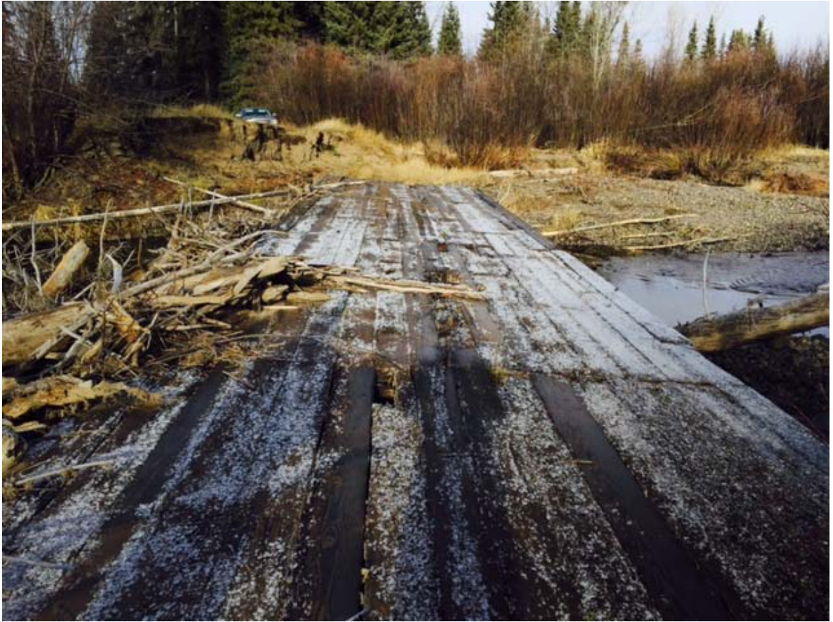
Photo 6. Decking and upstream debris, November 11, 2015.
