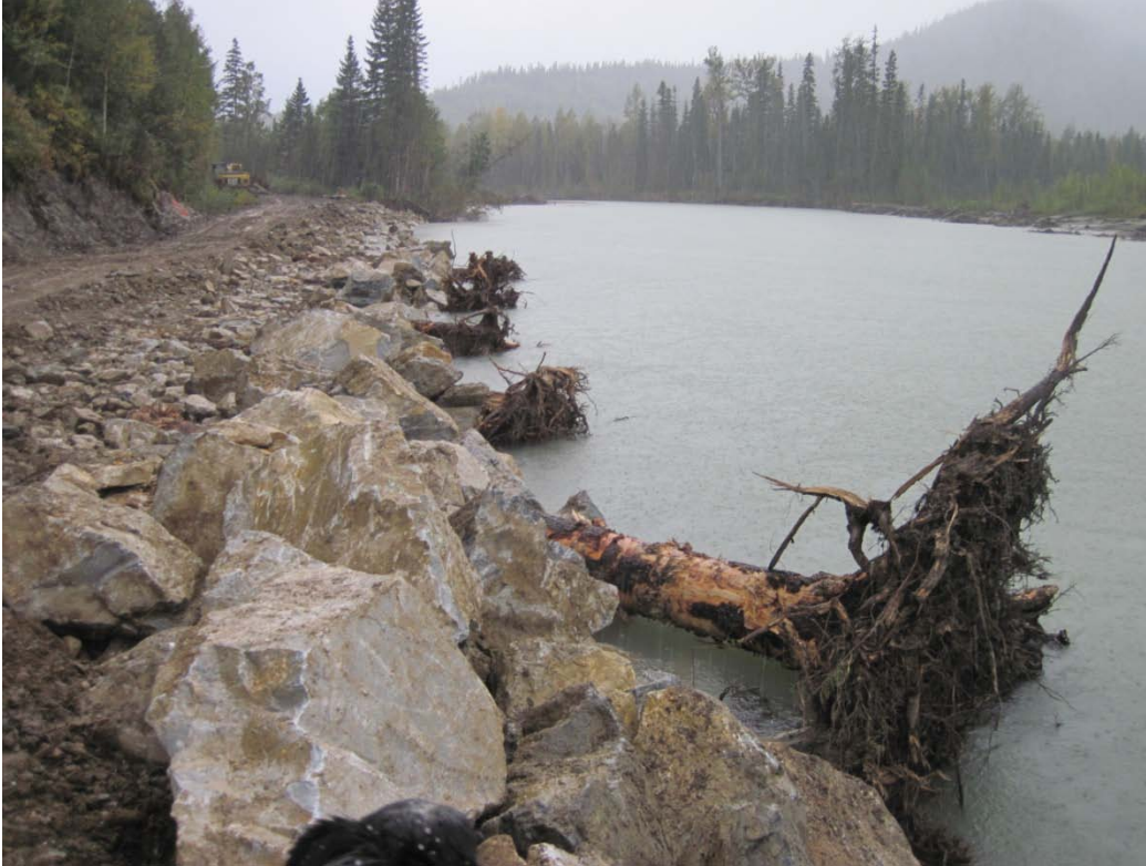
Photo 7. Examples of spruce logs with root wads which were obtained by pushing trees over with excavator.
