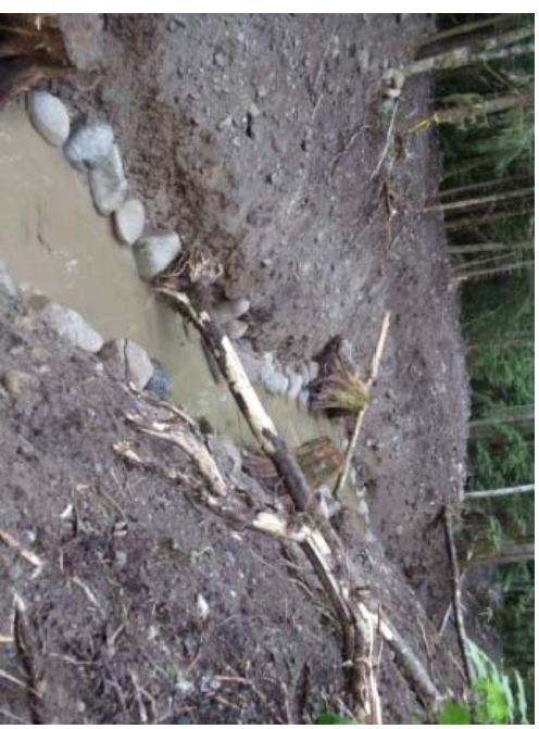
Photo showing typical excavation from Williams Creek 2011 including boulder placement and large woody debris (stumps)
