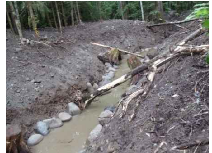
Photo showing Typical excavation from Williams Creek 2011 including boulder placement and large woody debris (stumps)
