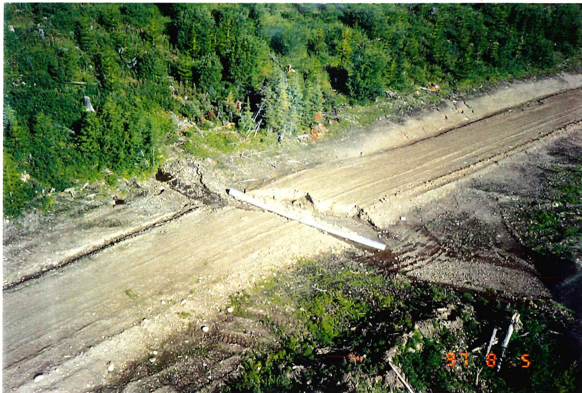
Pacman Lake tributary culvert failure
