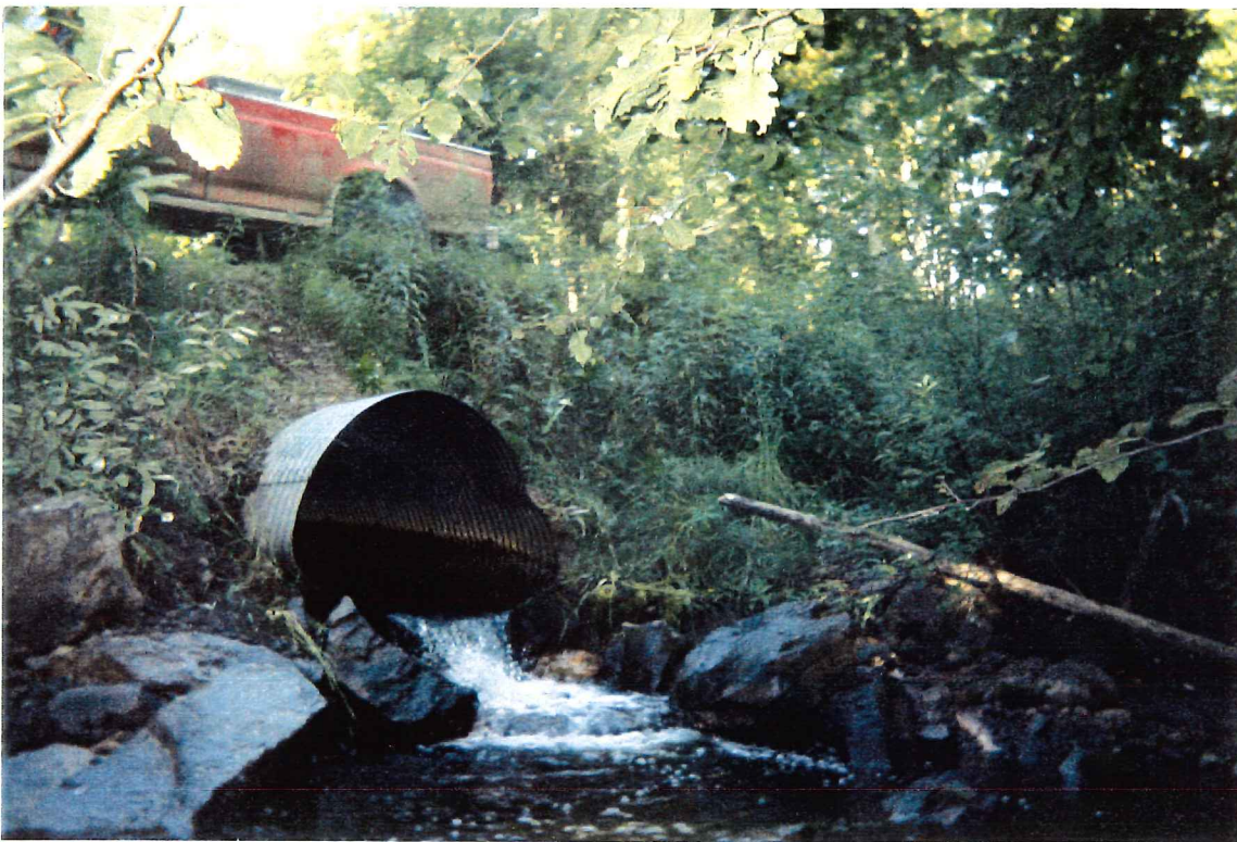
Cross Creek: Culvert is a barrier to fish passage
