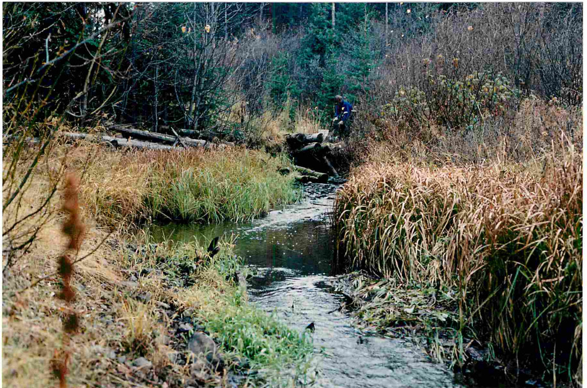
Figure 5. View upstream from McBrierie Lake inlet toward broken log bridge.
