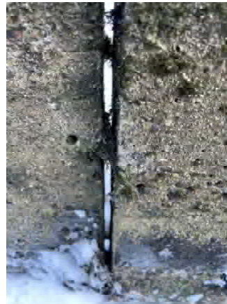
Photo 8 - Displacement between Boxes
