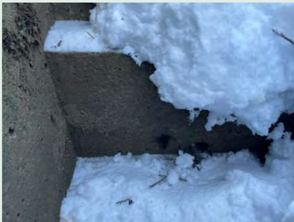
Photo 9 - Box Drain Hole
