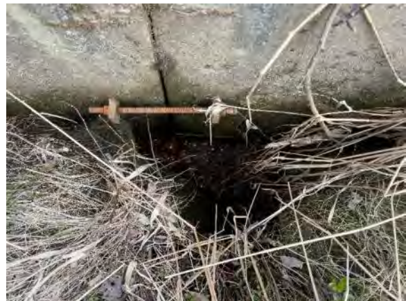
Photo 4 - Eroded Fill Adjacent to Boxes
