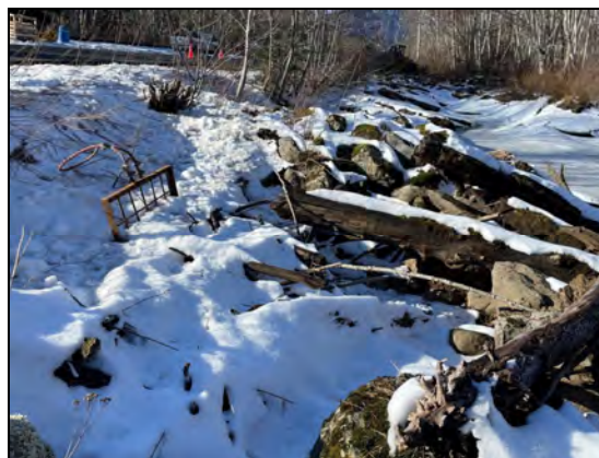
Photo 2 – upstream side of the highway, debris accumulated on the outlet pipe
