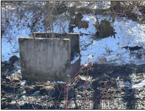
Photo 17 – component fishway box (Thomas)
