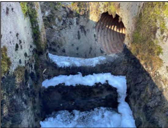
Photo 9 – corner box at the top of the fishway. Weir should be backwatering the culvert to the inlet
