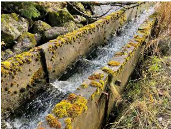
Photo 3 - Ladder View Depicting the Displacement
