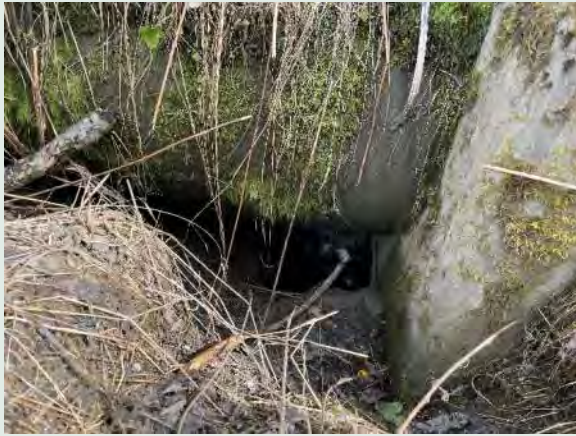
Photo 13 - Erosion under the pipe
