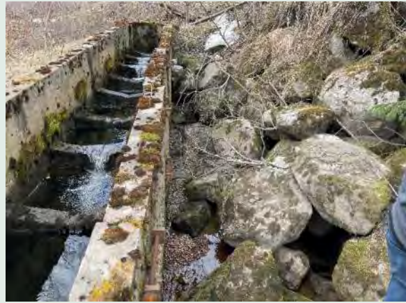
Photo 4 - Erosion between rail riprap and fishway
