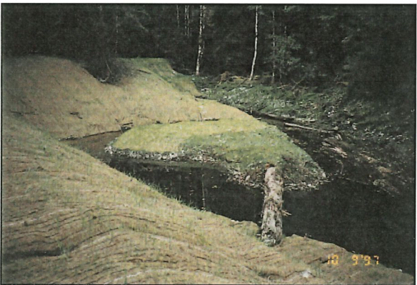
Figure 6-12. Upper end of King Creek "blind" side channel after placement of erosion control matting and grass seeding.
