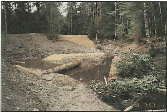
Figure 6-11. Upper end of King Creek "blind" side channel prior to laying of erosion control matting. Note construction of island to increase the irregularity of the channel margin.
