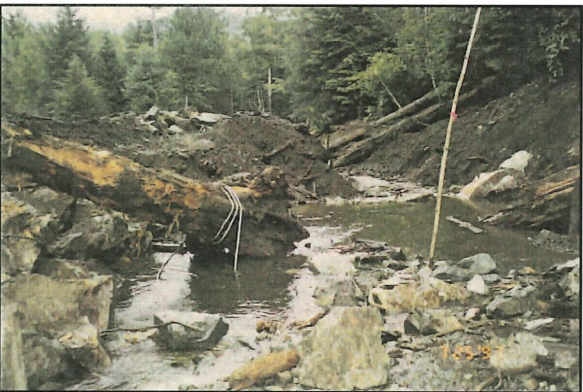
Figure 6-5. Initial placement of LWD in a partially constructed channel prior to reconnecting stream flows on Thurston Creek.
