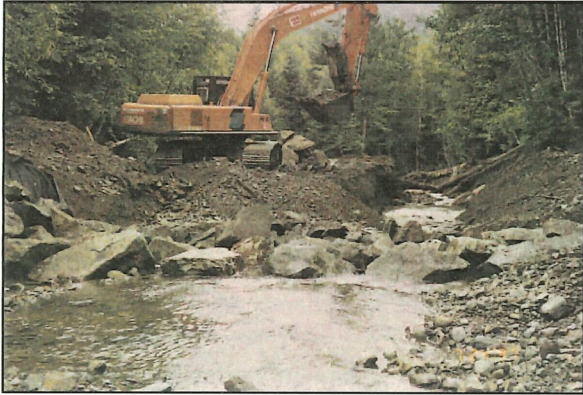
Figure 6-3. Latter stages of removing tormented material at the site of the diversion. This stage of work reconnected upper Thurston Creek with lower Thurston Creek after 10 to 20 years of de-watering.
