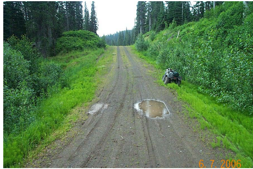
Figure 9. Crossing SB07-Surface water confined along wheel grooves puddles and spills into stream at culvert crossing.
