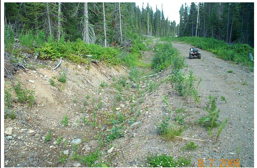
Figure 14. Crossing SB67-coarse material falling off cutslope is trapped by several small retention features
