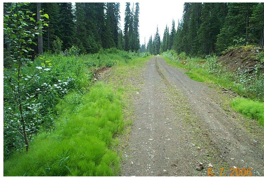
Figure 13. Crossing SB03-small ditch-line remains active sediment source.
