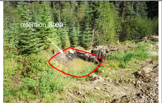
Medium Sized retention area re-enforced with geo-textile to minimize erosion when structure overfills.
