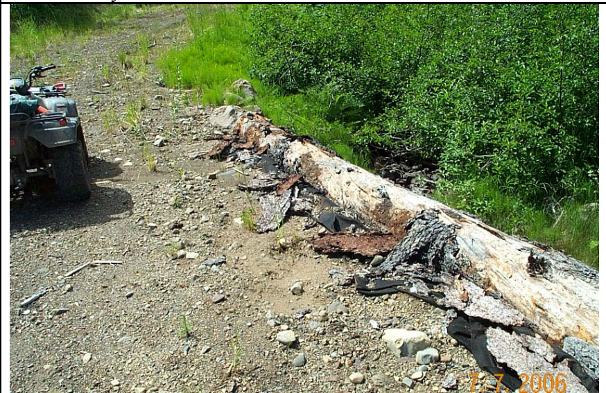
Figure 8. Crossing SB27-Coarse sediment trapped on bridge but fine sediments spill directly into stream.
