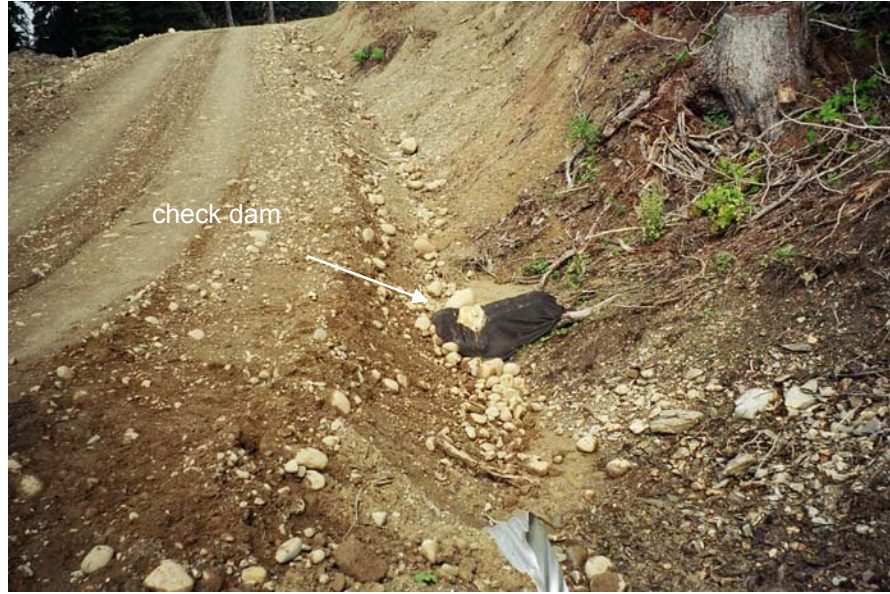
One check dam located along sediment source 10-40% up from stream (Location score = 0.85).
