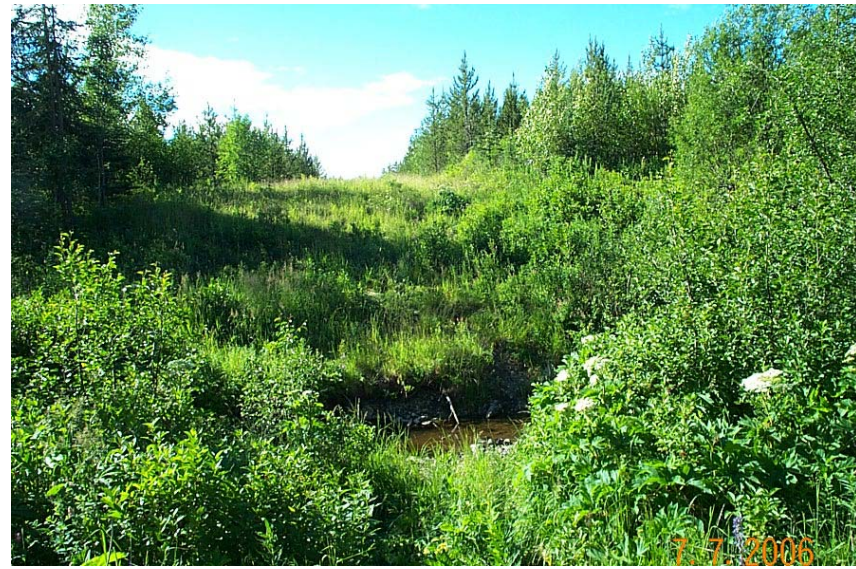
Figure 17. Crossing SB32- road surface and ditches completely covered by vegetation
