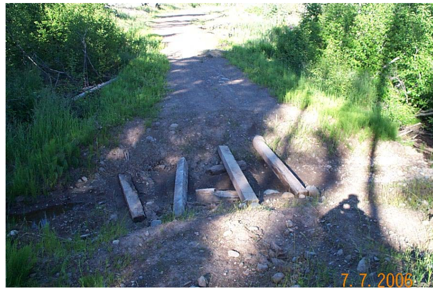
Figure 11. Crossing SC33- approaches left after culvert removal require vegetation or protection from raindrop erosion.
