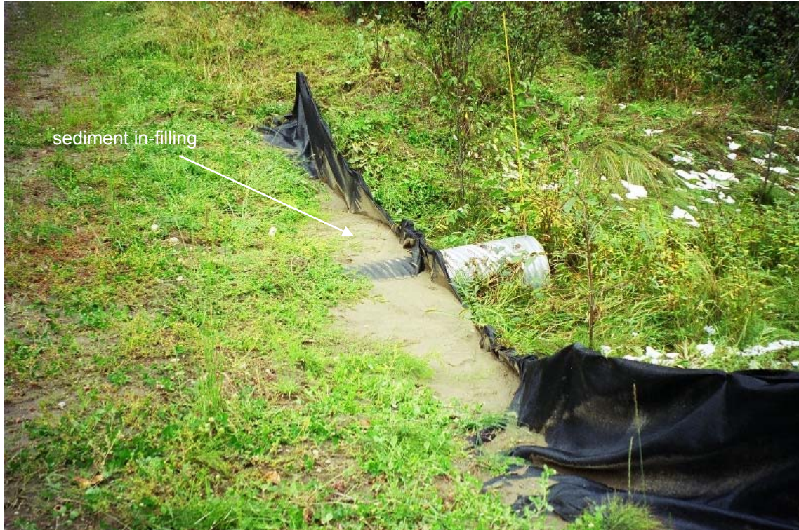
Figure A1-5 Sediment pond with nearly 100% in-filling has virtual no capacity to retain sediment. Using Table A1-8, the net size is “Very Small”.
