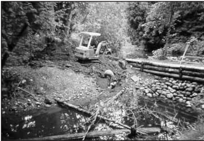
Figure 6-15. Additional culvert intake installed to increase low flow levels in the side channel.
