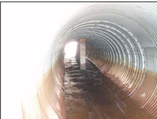
Figure 50. Glass Creek culvert interior. View upstream from culvert outlet showing support beams.
