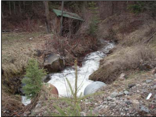
Figure 59. Tyhee Creek culvert outlets. View downstream to outlets in high water, spring, 2007.
