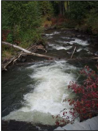
Figure 24. View of Toboggan Creek culvert downstream. Photo shows low flow conditions September 21, 2006.
