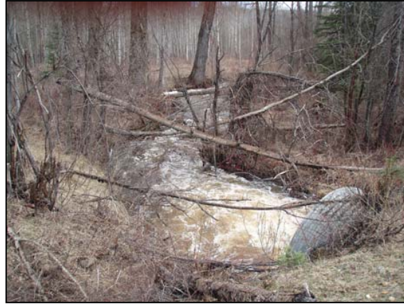
Figure 69. Coffin Creek culvert outlet. View downstream of outlet in high flow conditions.
