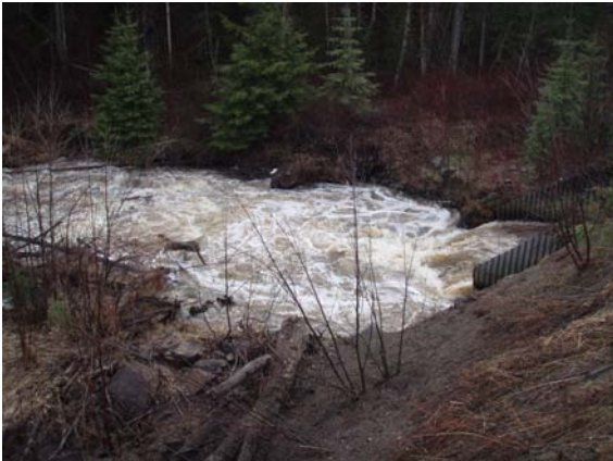
Figure 27. View of Toboggan Creek culvert outlet. Photo shows high flow conditions May 04, 2007.
