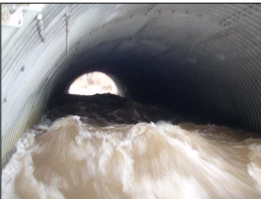
Figure 29. View of Toboggan Creek culvert inside. Photo shows high flow conditions May 04, 2007. Culvert water velocity averaged 3.37 m/s.
