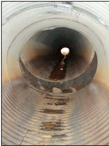
Figure 54. McDowell Creek culvert. View upstream from culvert outlet to separated joint.
