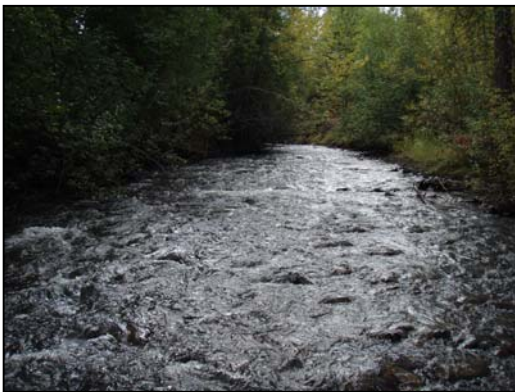
Figure 25. View of Toboggan Creek culvert upstream. Photo shows low flow conditions September 21, 2006.
