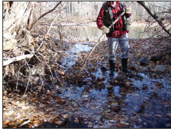
Figure 38. Moan Creek culvert outlet. View downstream from culvert outlet with Bulkley River in the background.
