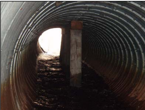
Figure 49. Glass Creek culvert interior. View downstream from culvert inlet showing sag and support beams.
