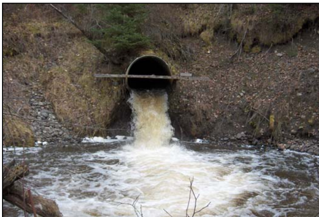
Figure 7. Station Creek culvert with a 1.5 m outfall drop. This culvert passing under Highway 16 does not allow fish passage.
