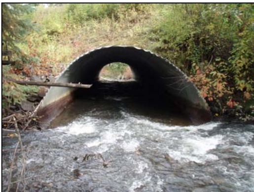
Figure 26. View of Toboggan Creek culvert inlet downstream. Photo shows low flow conditions September 21, 2006.
