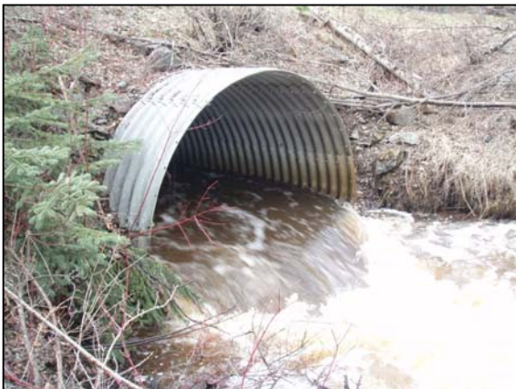
Figure 67. Coffin Creek culvert outlet. View upstream of outlet in high flow conditions.
