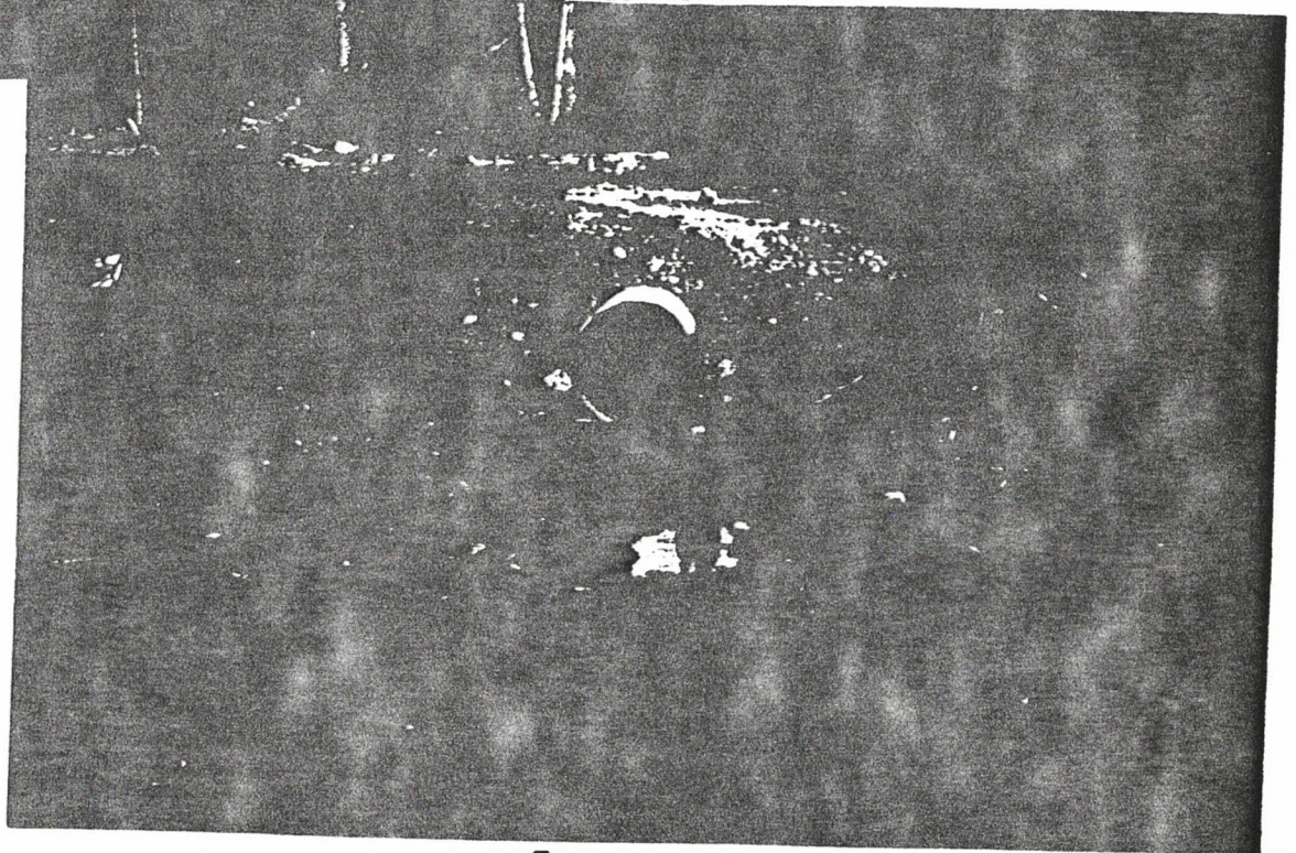
Figure 3 (Below). Creek 460-6006-364-263 Site C. Damage due to recent road construction. Note turbidity of water, lack of riparian vegetation and vegetation on banks of road, soft substrate immediately downstream of culvert.
