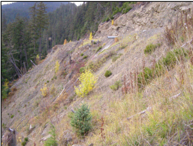
Figure 115. View westward across slide located 340 m downstream of the bridge crossing West Kitsuns Creek. Note over-extended perched culvert delivering drainage to unstable slope.
