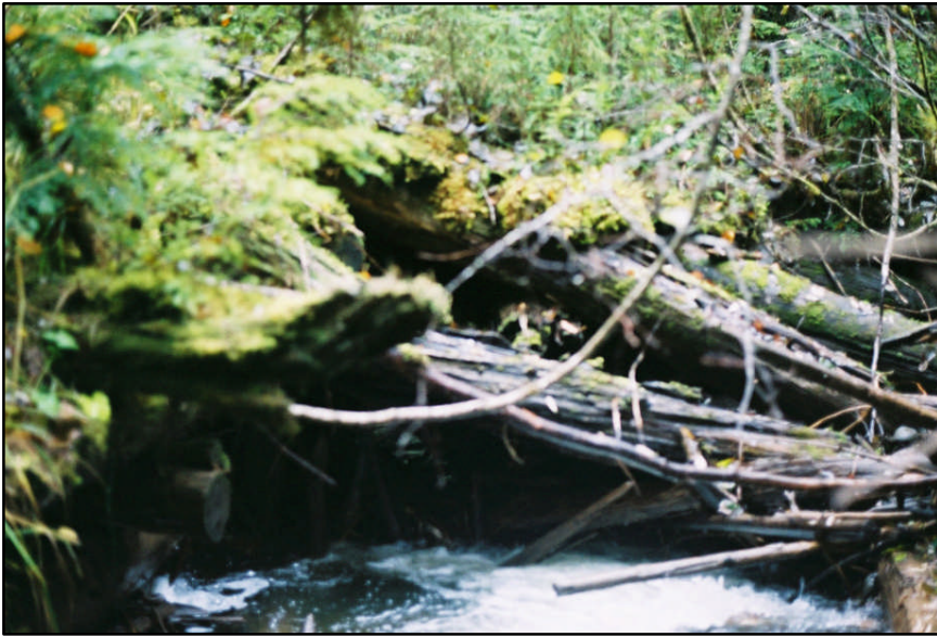
Figure 96. Close view downstream of collapsed structures Fifteen Mile Creek.
