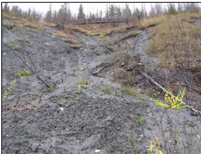
Figure 77 . Wasting in Area #4.
