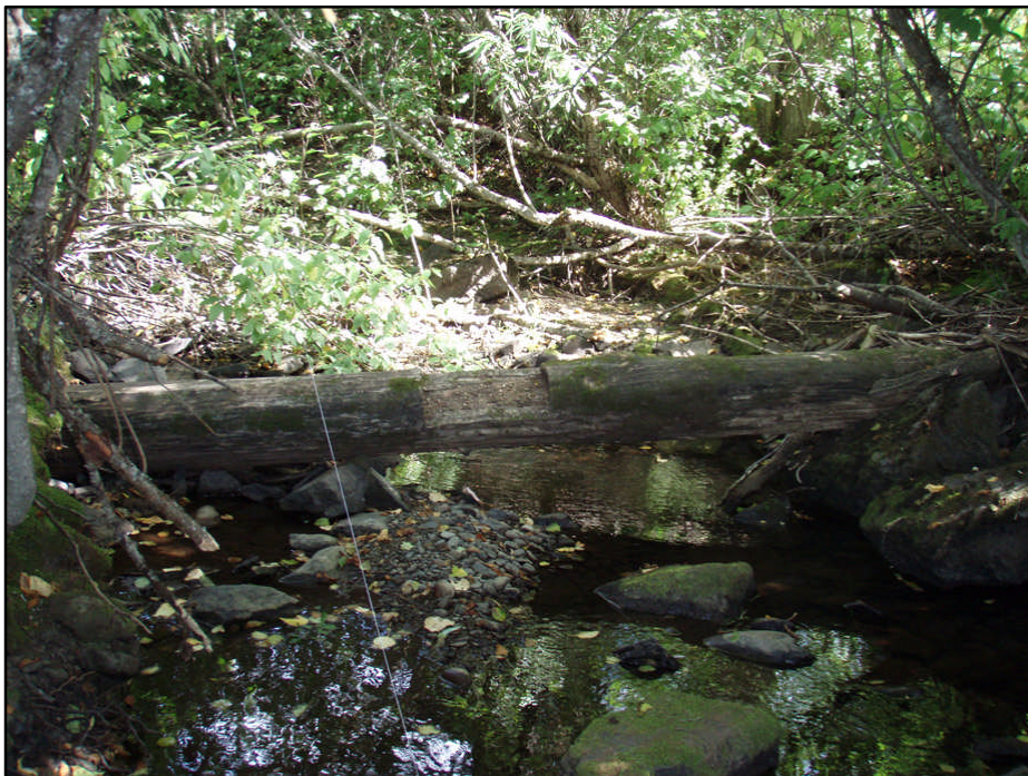
Figure 5. Notched weir log 15 m downstream of culvert. 40 cm log was installed in 1997 to increase height of outfall drop pool.
