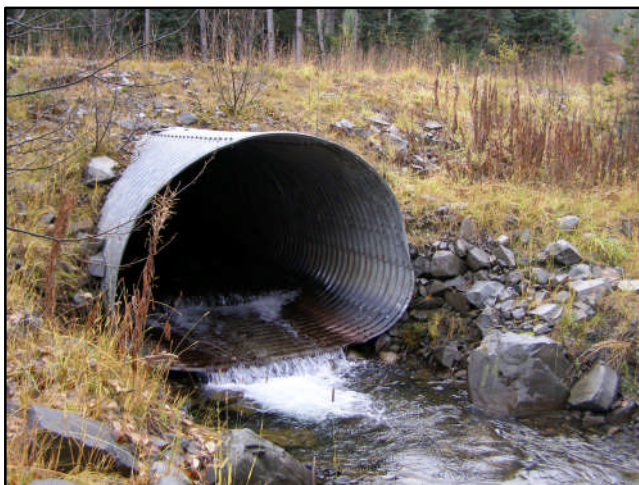
Figure 94. Side view shows 17 cm culvert outfall drop.
