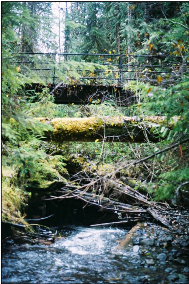
Figure 95. View downstream of collapsed structures.
