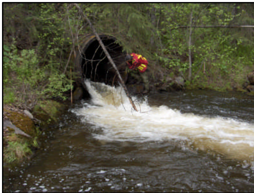
Figure 53. Skunsnat Creek culvert outlet. View of outlet from downstream with velocities over 3.1 m/s.
