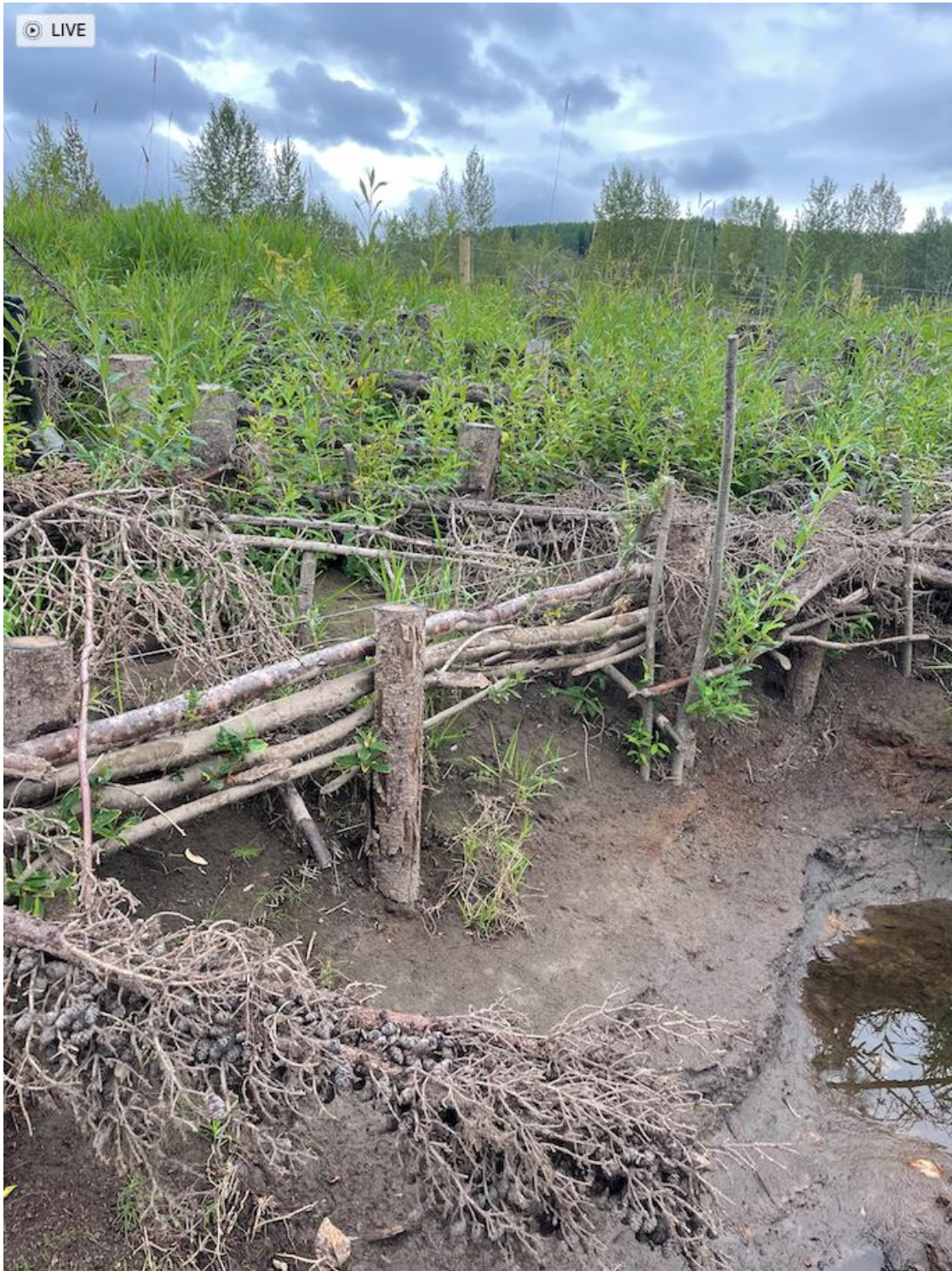
Figure 2: Photo showing undercutting at Dickson site.
