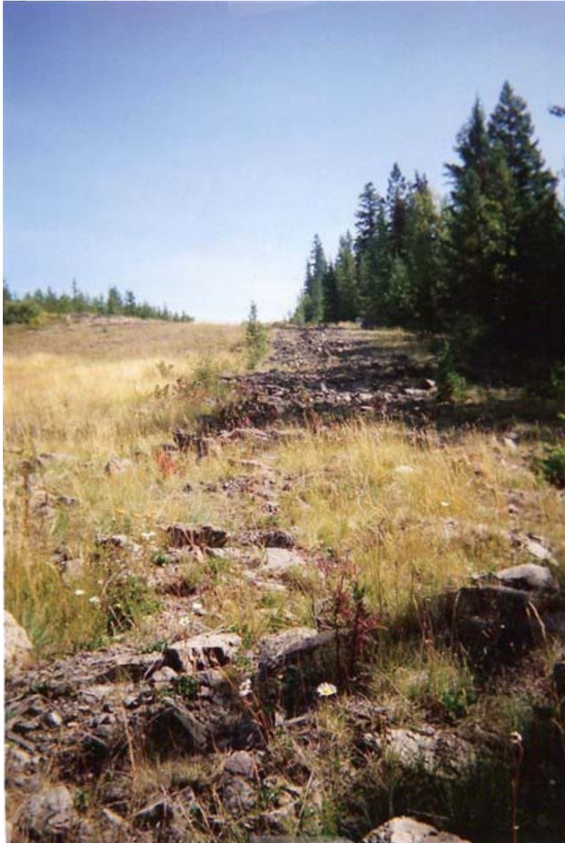
Photo 5 Consolidated bedrock was encountered at shallow depths during construction of the previous pipeline. Such an area is mapped as Rock (R) soils. Site 68 at KP 327.4.
