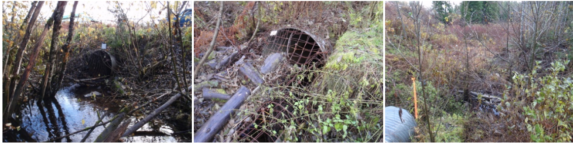
Figure 11 Crossing structure 377977 on Kozier Rd., the culvert outlet (left), inlet (middle), and upstream (right).
