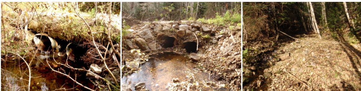
Figure 4. Crossing structure EX007, the culvert outlets (left) and inlets (middle) and upstream (right).
