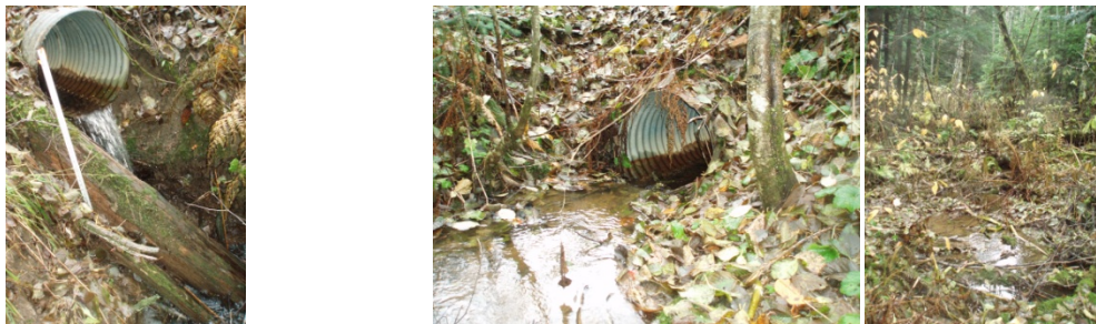
Figure 13 Crossing structure AL002 on Matson Rd., the culvert outlet (left), inlet (middle), and upstream (right).
