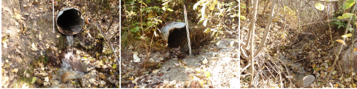
Figure 9 Crossing structure 377970, the culvert outlet (left) and inlet (middle) and upstream (right).
