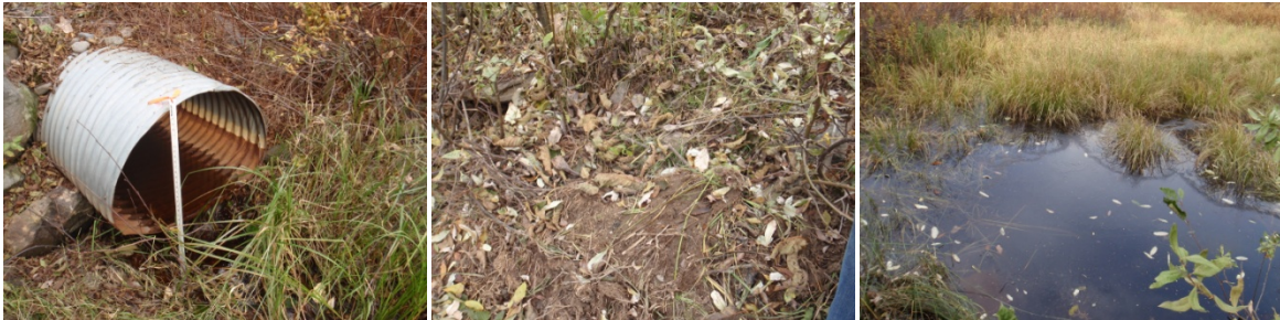
Figure 3 Crossing structure EX005, the culvert outlet (left) and inlet (middle) and upstream (right).
