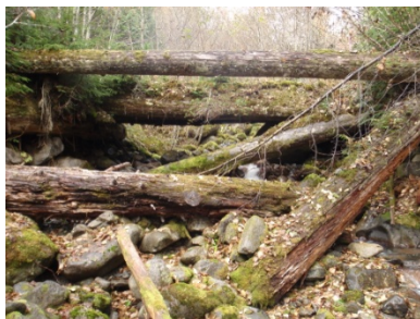
Figure 16 Old collapsing bridge across Delta Creek (crossing structure 378065)
