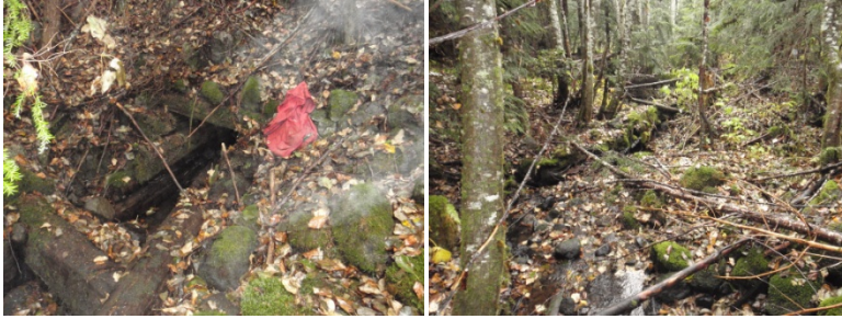
Figure 17. Collapsing WBC creating a 1 meter fish barrier (left) and upstream habitat (right). Crossing structure 377976 on unnamed creek east of Amsbury Creek.
