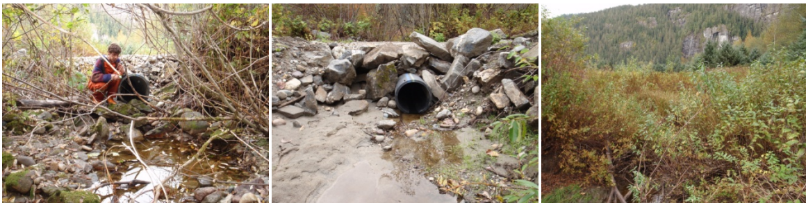
Figure 5. Crossing structure 377319, the culvert outlet (left) and inlet (middle) and upstream (right).
