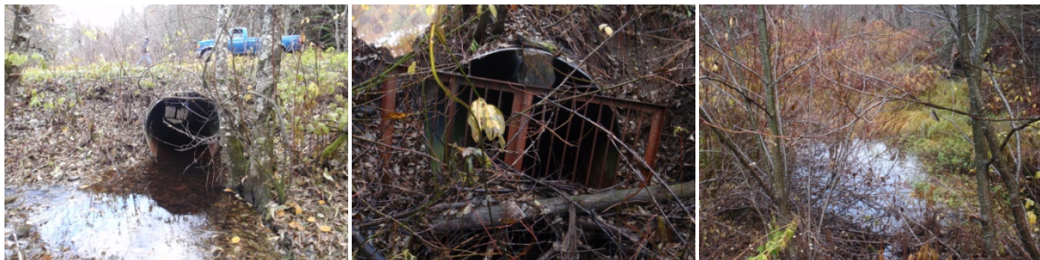
Figure 14 Crossing structure 377968 on Old Remo Rd., the culvert outlet (left), inlet (middle), and upstream (right).
