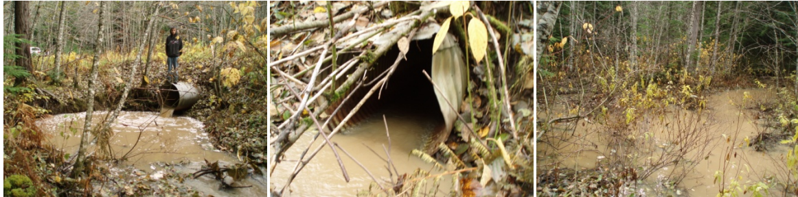
Figure 12 Crossing structure 378039 on Matson Rd., the culvert outlet (left), inlet (middle), and upstream (right).
