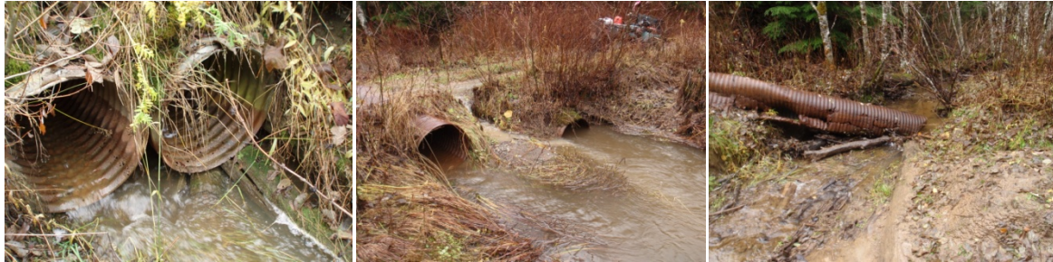
Figure 15. Crossing structures along the hydro line which should be removed or replaced with OBS. (378044 is shown on the left, 378019 is in middle and 378034 is shown on the right).
