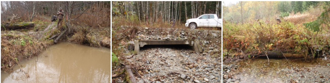
Figure 18 WBC in poor condition. Crossing 378021 (left), DAS010 (middle) and WB006 (right). DAS010 and WB006 are nearly blocked with alluvial deposits resulting in poor fish passage conditions.
