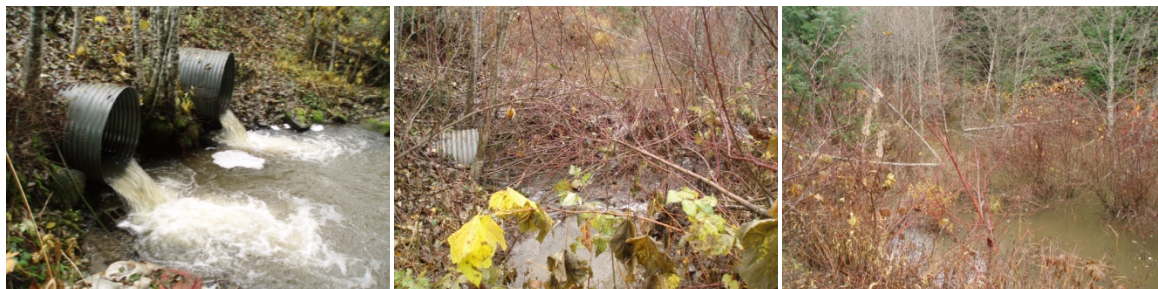
Figure 10 Crossing structure 378014 on Matson Rd., the culvert outlets (left), inlets and beaver dam (middle), and upstream (right).
