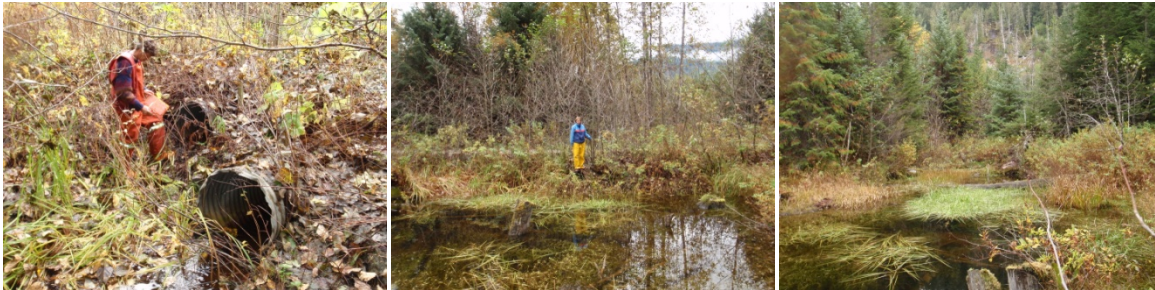
Figure 7 Crossing structure 377279, the culvert outlets (left) and inlets (middle) and upstream (right).
