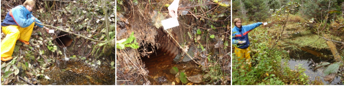
Figure 6. Crossing structure 377276, the culvert outlet (left) and inlet (middle) and upstream (right).
