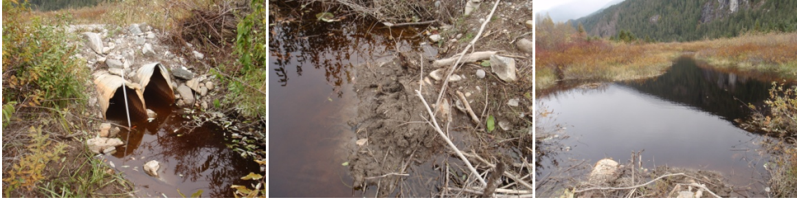
Figure 2. Crossing structure EX004, the culvert outlets (left) and inlets (middle) and upstream (right).
