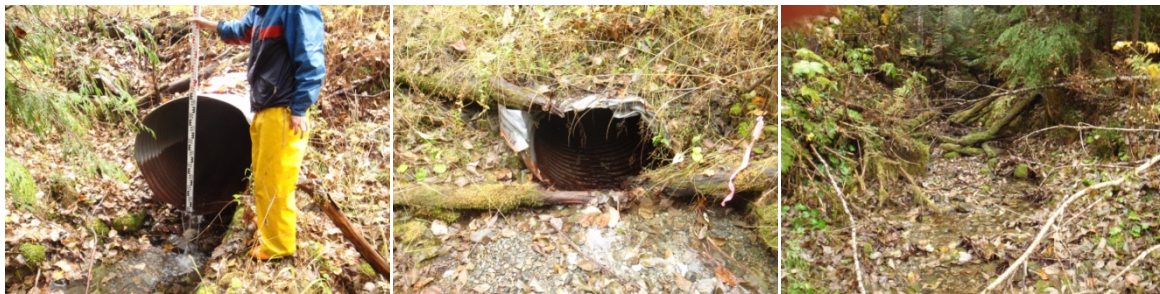
Figure 8 Crossing structure 377334, the culvert outlet (left) and inlet (middle) and upstream (right).
