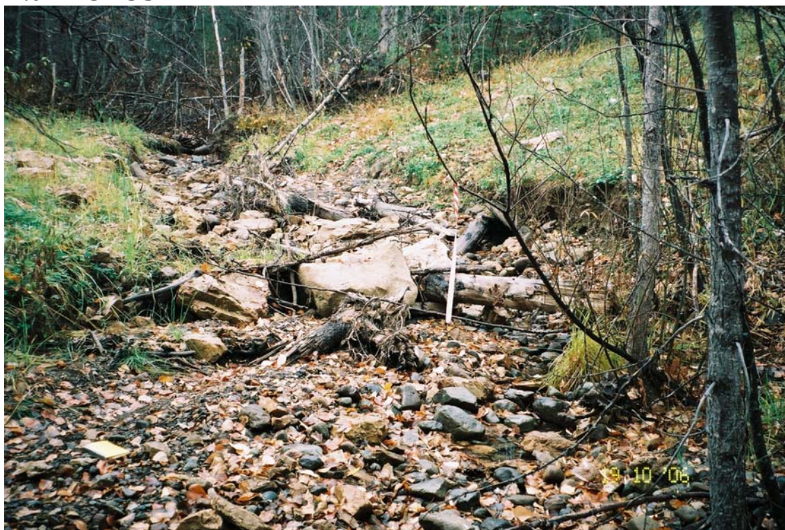
Site 3006-1. Upstream view of reconstructed channel. Note bank scour at toe of loaded approach to right of ribbon.
