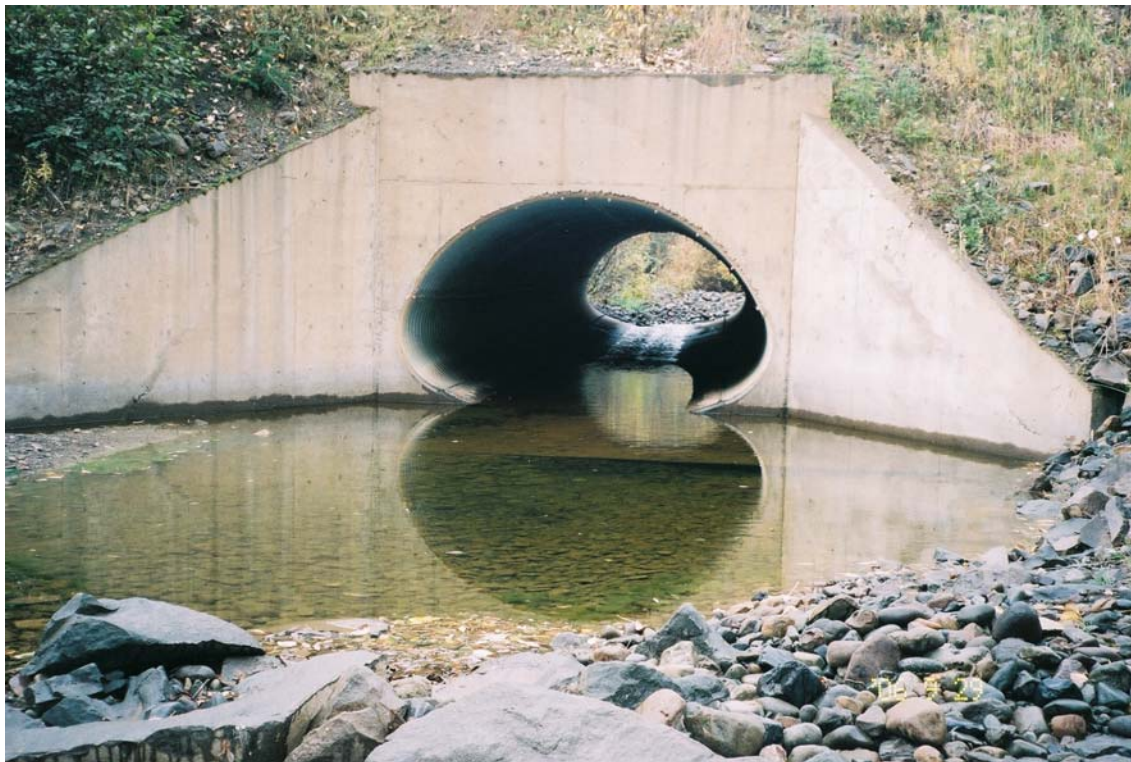
Site 4000-Feature 17/678. Williams Creek. Upstream view of backwatered culvert outlet, in-filled outlet pool.
