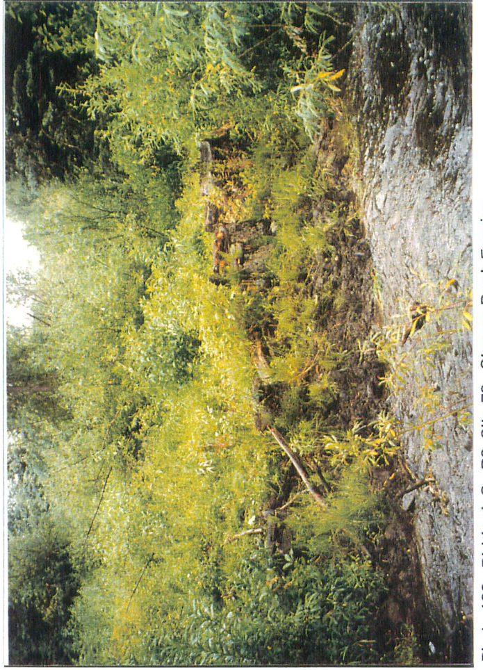
Photo 188. Riddeck C., R2, Site 79 - Stream Bank Erosion
