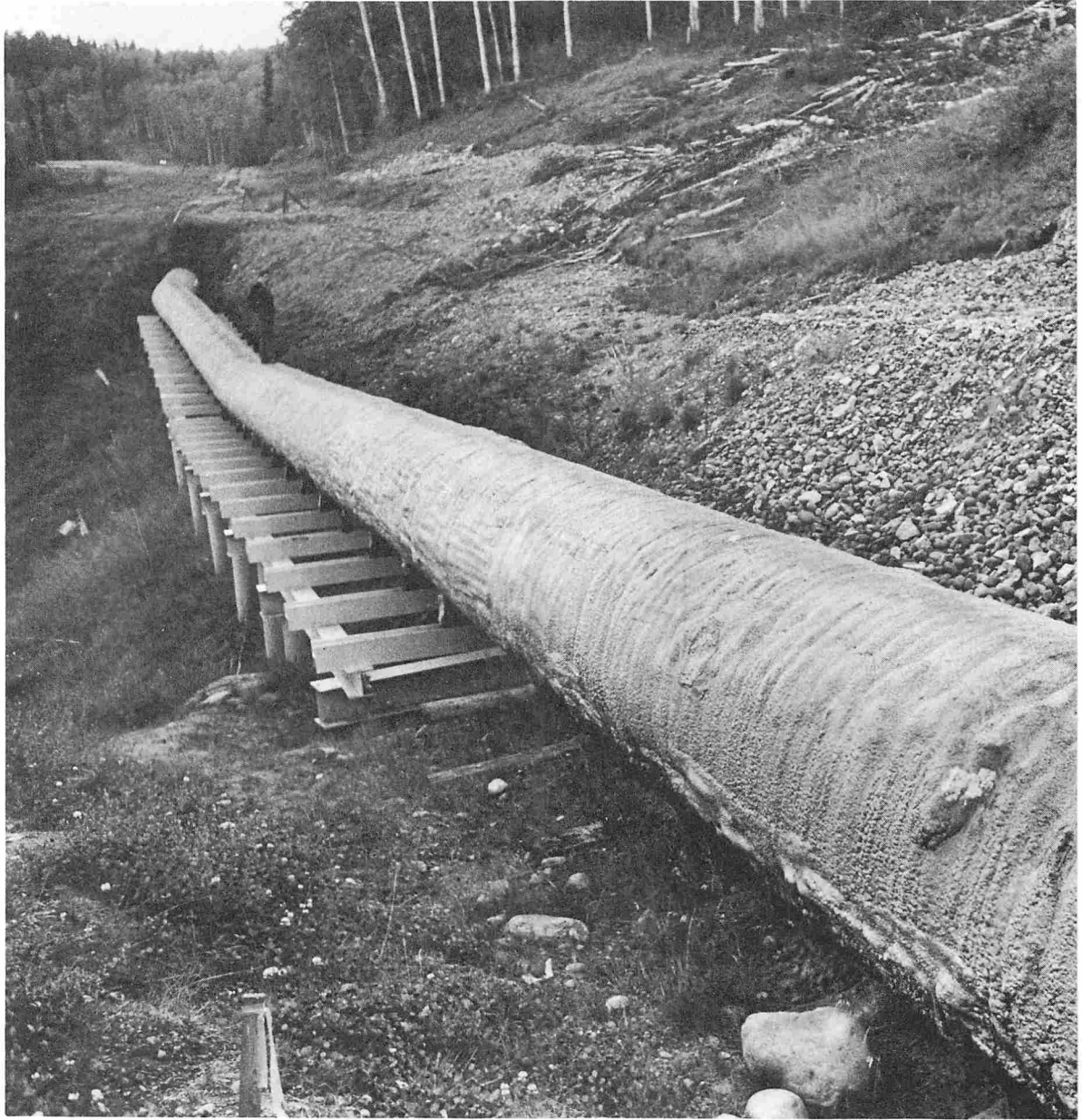
Figure 6: Exposed section of water supply pipeline to Fulton River Spawning Channel No. 2.
