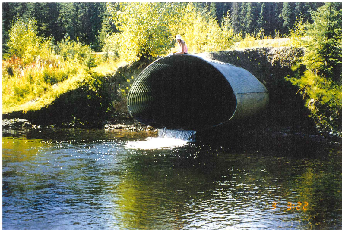
Plate 56: Culvert on McQuarrie Creek at the North Road FSR. This culvert may be a barrier to fish migration due to water levels and velocities, as well as length. It will definitely become more of a problem as height from the water surface to the culvert inlet increases due to downcutting. Note the already extensive erosion.
