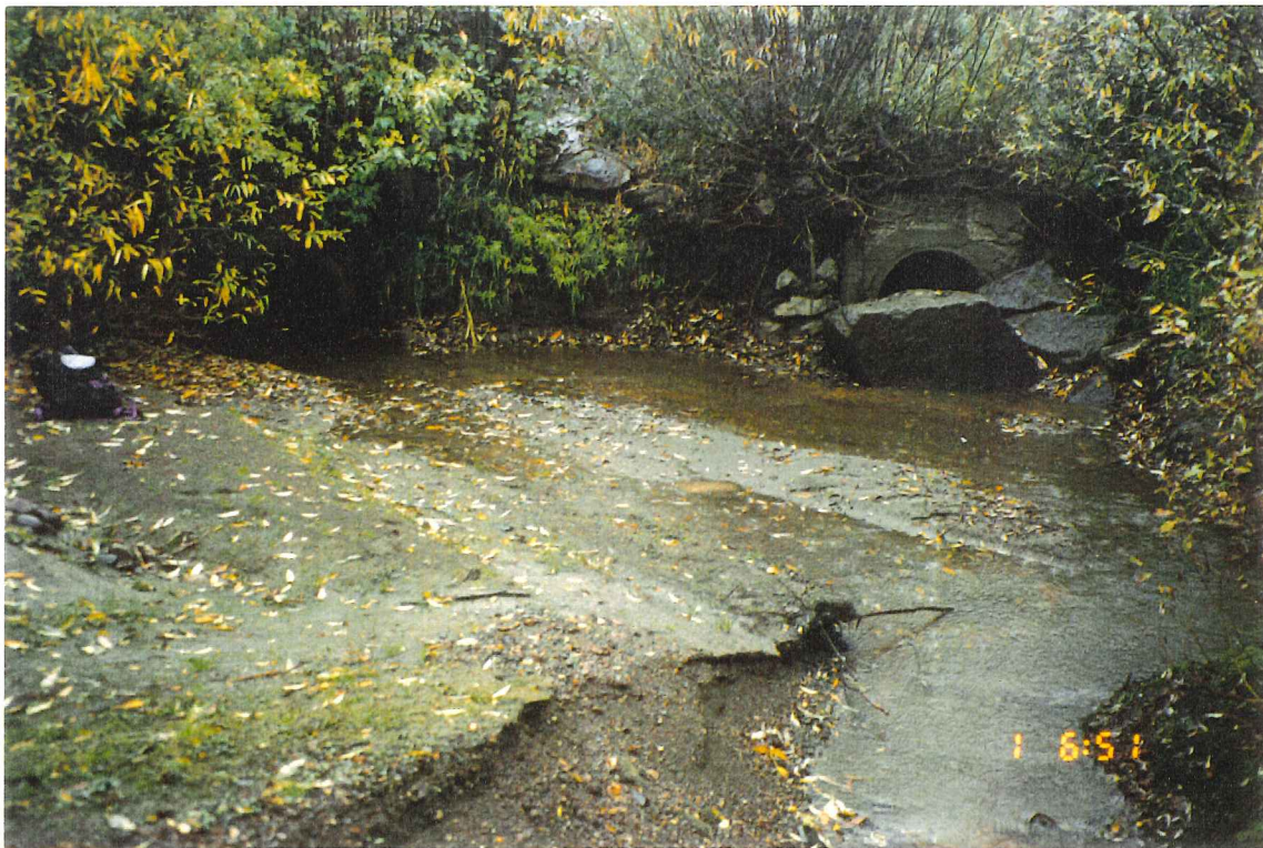
Plate 58: Barren Creek at the Bulkley River. Note that the mouth is heavily aggraded with fine material and one culvert is blocked in the background. These concrete culverts at the CN Rail crossing are very smooth and consequently water velocities will be high. They are also probably too undersized to facilitate fish passage in even normal bankfull flood events.
