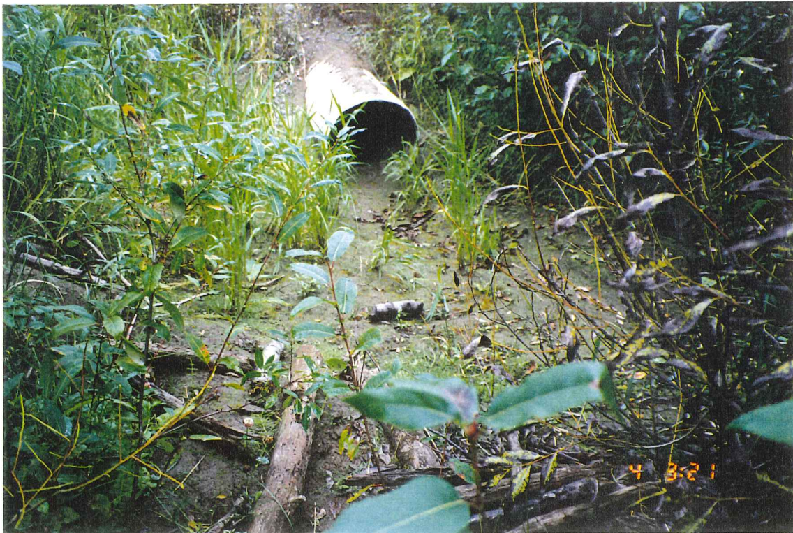
Plate 52: Blocked culvert to downstream end of offchannel area on Byman Creek. The other side of the culvert is high and dry.
