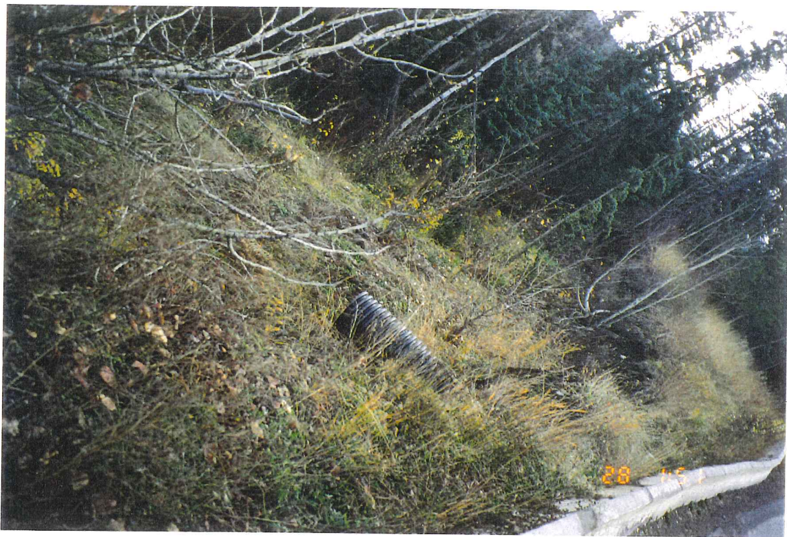
Plate 19: Slide scarp of large rotational slump above Buck Creek, Reach 1C. The slump is occurring at the edge of a suburban road along the lip of the slope. It shows high connectivity to the active channel of Buck Creek.
