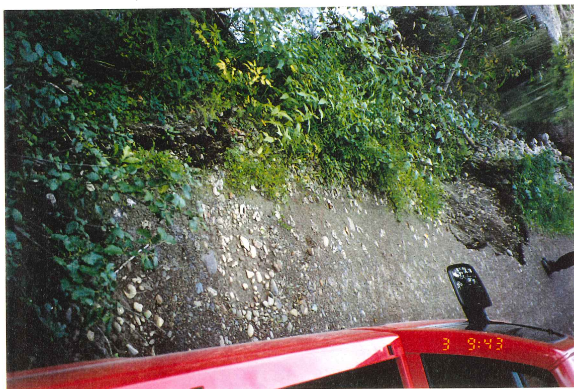
Plate 24: Road adjacent to Buck Creek in Reach 4B eroding directly into creek.
