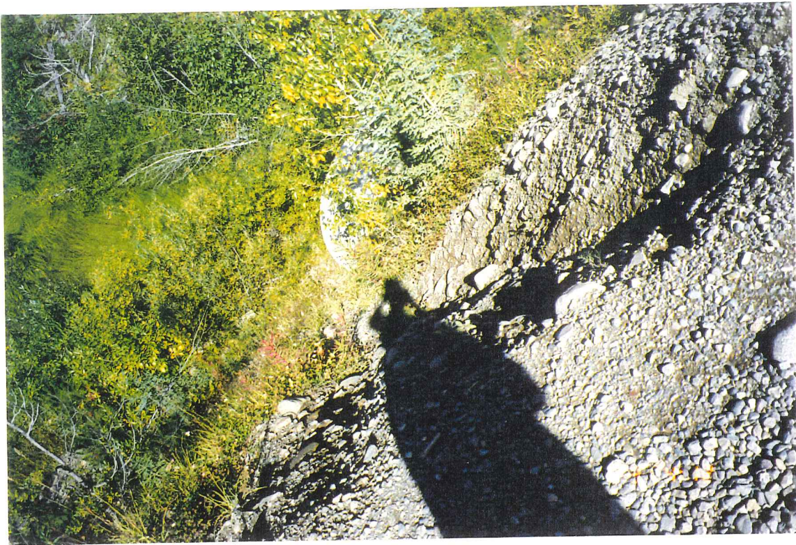
Plate 49: Extensive erosion of the North Road FSR fill slope into an intermittent Unnamed tributary to Johnny David Creek. The fill slope is eroding on both sides of the crossing due to use of relatively fine-textured fill.
