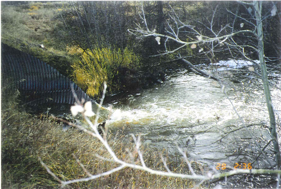
Plate 51: Culvert at highway crossing on Byman Creek. This culvert appears to be passable as a function of height above the water surface, length, diameter, and gradient. It is suspected to be a barrier due to water velocities at high flows and water levels at low flows.
