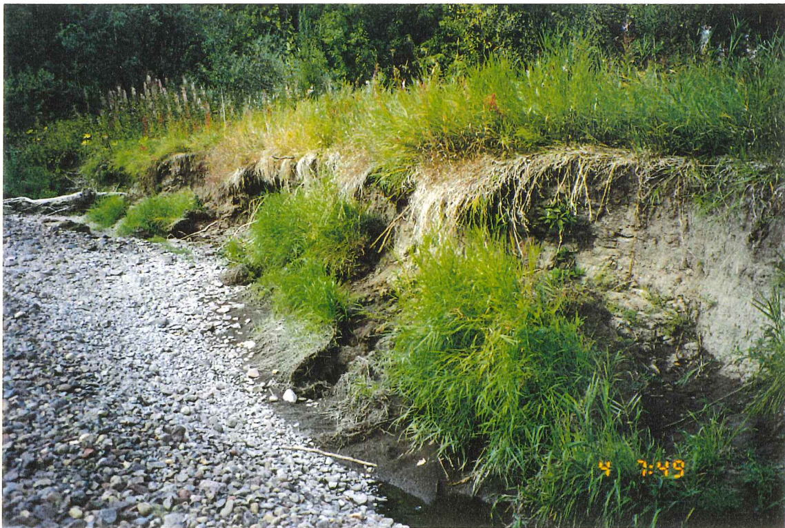
Plate 16: Extensive bank erosion downstream of the channelized section of Buck Creek (Reach 1B).
