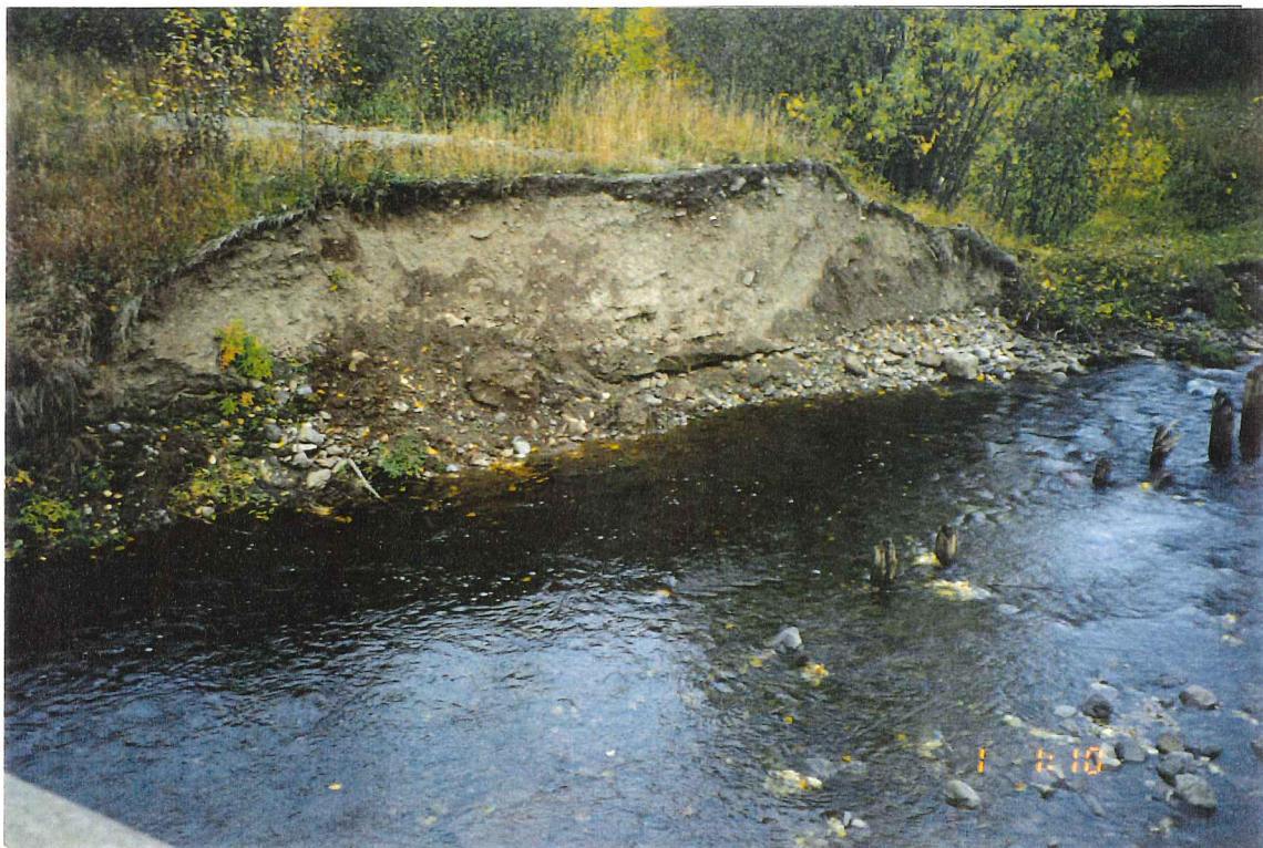
Plate 26: Old bridge abutment at the second Buck Flats Road bridge is wasting into the creek.
