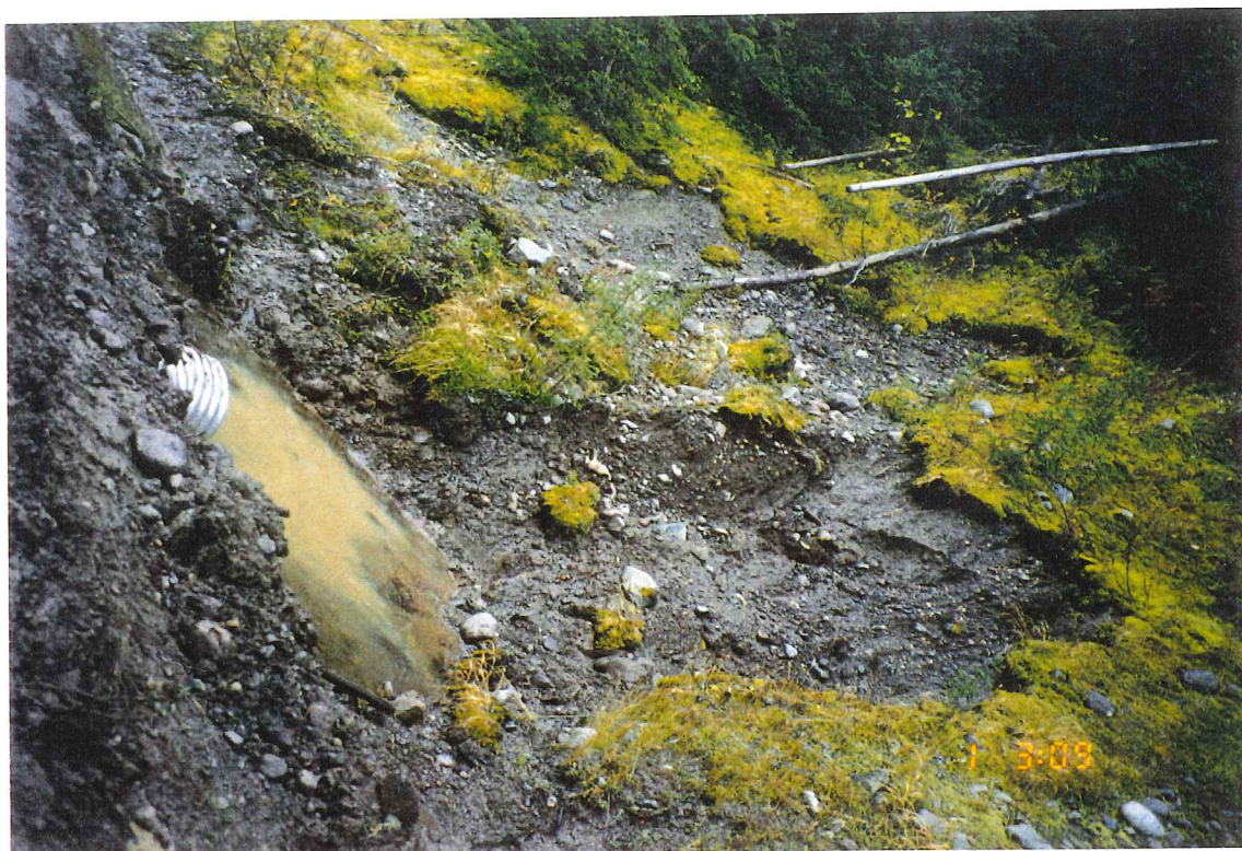
Plate 33: Failing slope above culvert on FSR is a source of fines to Upper Buck Creek, Reach 11B.
