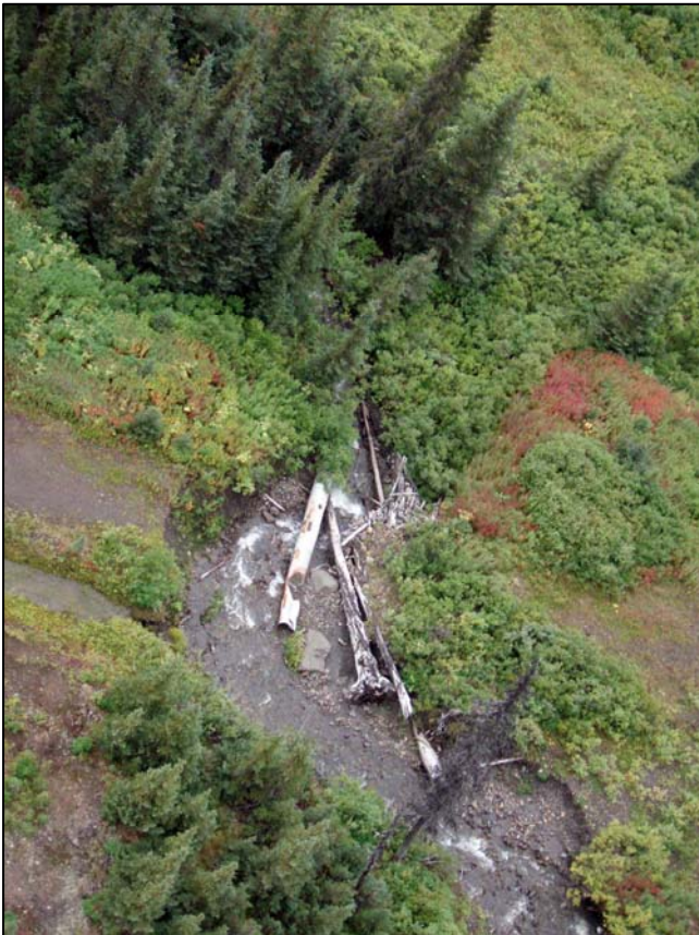
Figure 72. Site 120, washed out culvert on Unnamed Creek.
