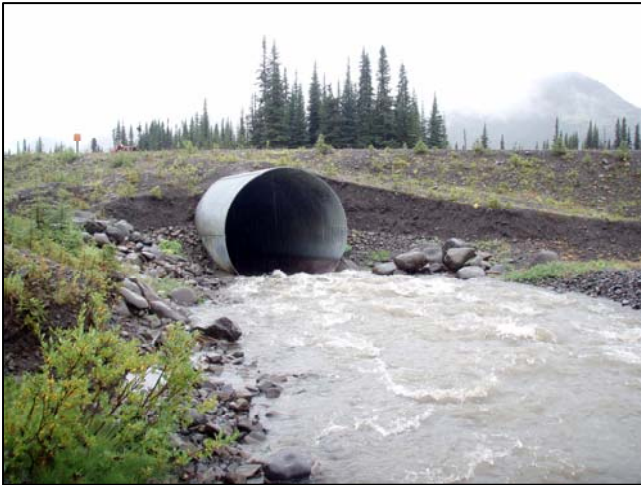
Figure 58. View downstream to Garner Creek culvert inlet. Note the erosion of the grade fill.
