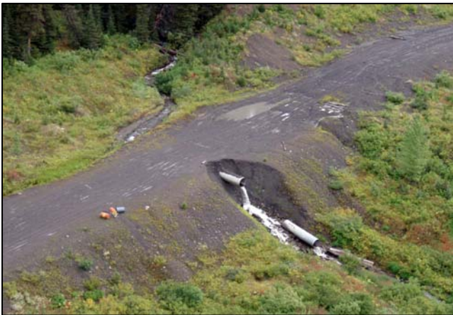
Figure 70. Site 86, Unnamed Creek. View shows washed out culvert outlet.
