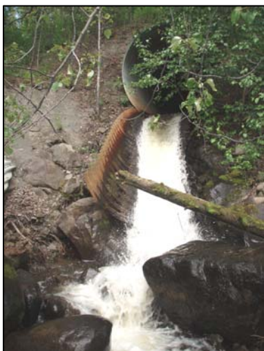
Figure 2. Photo shows culvert outlet flow down trough that establishes a definite fish passage barrier due to gradient and velocity issues.
