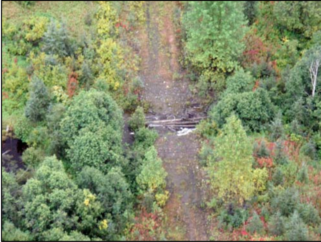
Figure 61. Site 56, Telfer Creek and washed out culvert.
