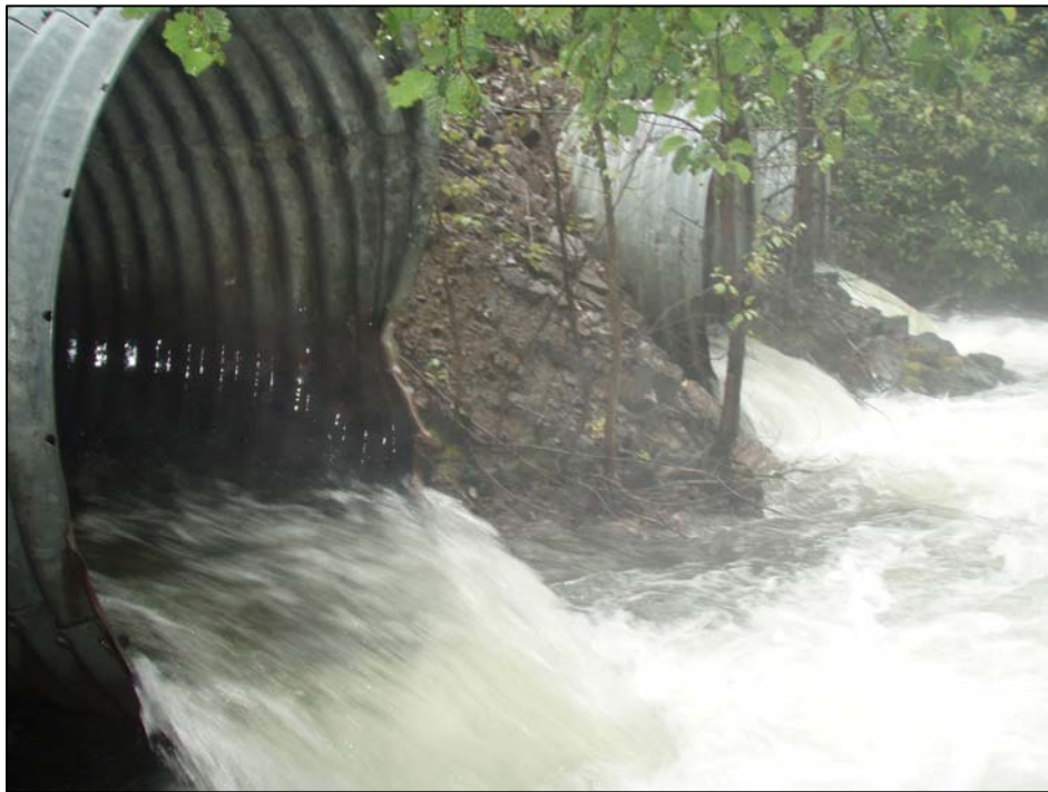
Figure 4. Typical B.C. Rail — three culvert installation on a high fish value crossing. The high water velocity and outfall drops constitute a fish passage barrier.
