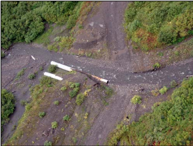
Figure 71. Site 91, view shows washed out culverts.
