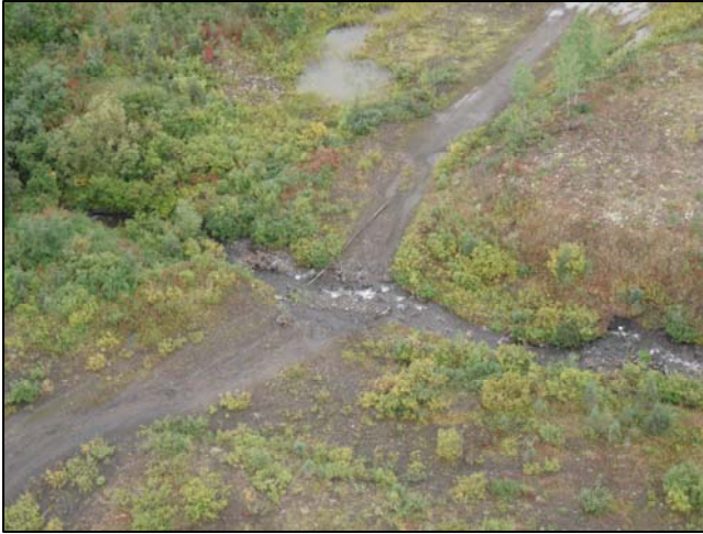
Figure 67. Site 69, view shows washed out culvert.
