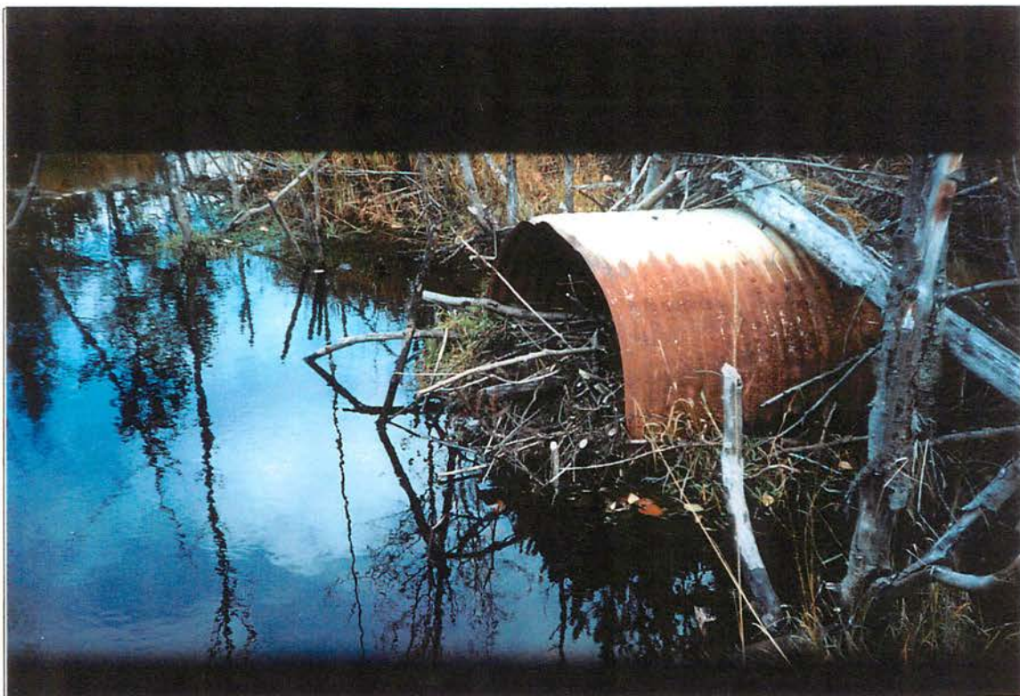
Site #375, Upstream photo of 0.6 m culvert plugged by beavers. Roll #79, Frame #01, Date: 2002/10/08
