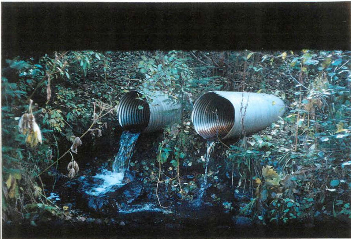
Site #367, Upstream photo of two perched culverts. Roll #80, Frame #10, Date: 2002/10/07
