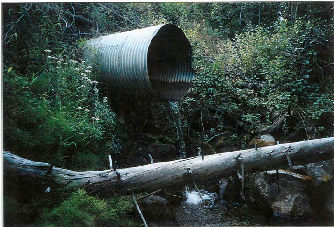
Site #8, Perched culvert - full barrier. Roll #1, Frame #19A, Date: 2002/08/27
