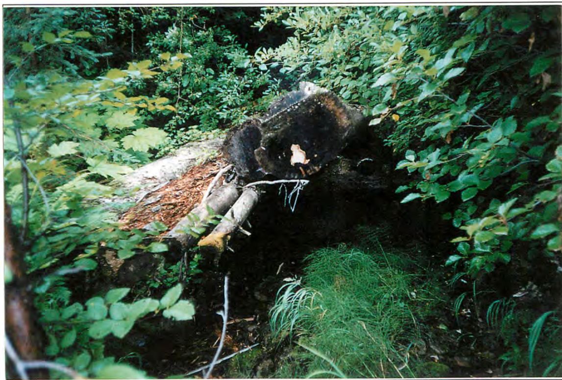
Site #13, Wooden box culvert in poor repair. Roll #2, Frame #1A, Date: 2002/08/28
