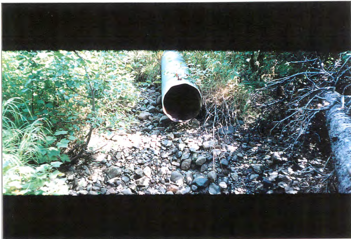
Site #27, Photo of eroded and perched culvert. Roll #3, Frame #11, Date: 2002/08/29
