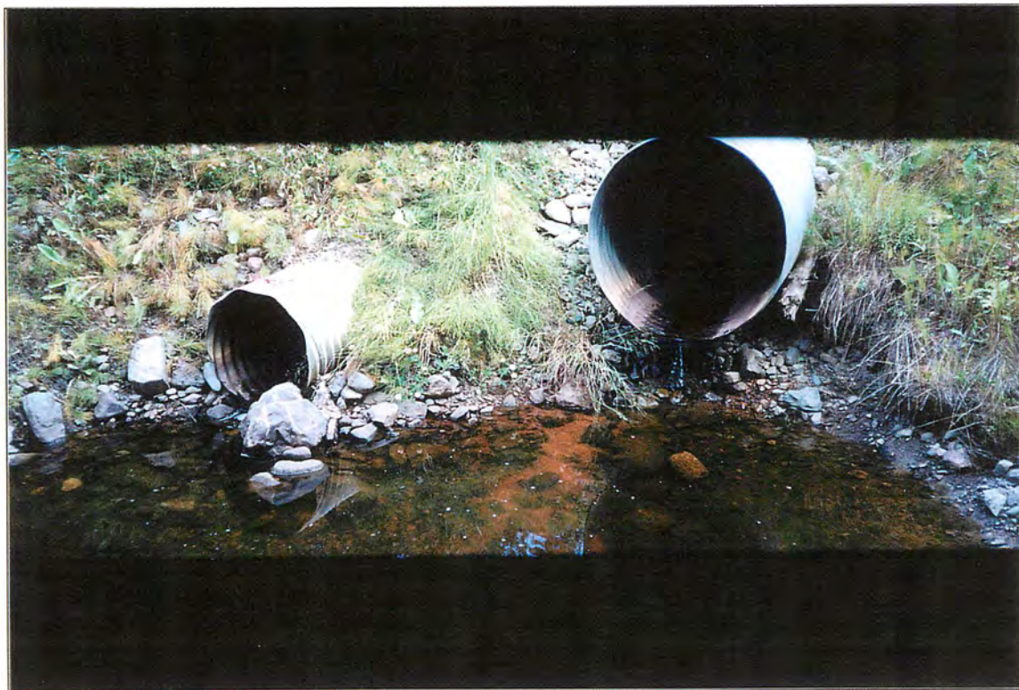
Site #28, Perched Culverts. Roll #3, Frame #16, Date: 2002/08/29
