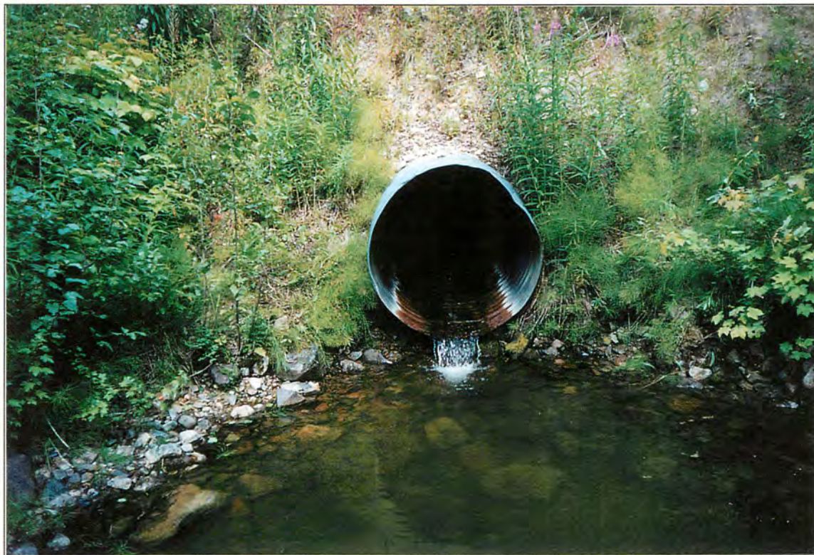
Site #7, Perched culvert, barrier to fish passage. Roll #1, Frame #14A, Date: 2002/05/27
