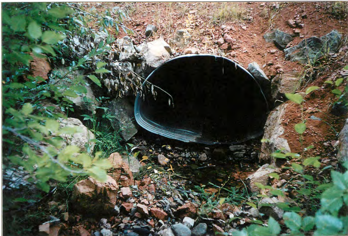
Site #13, Perched culvert in Reach 1 - partial barrier. Roll #1, Frame #23A, Date: 2002/08/28
