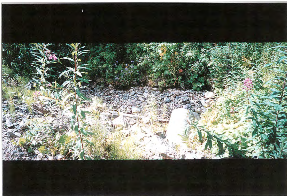
Site #27, Photo of eroded culvert. Roll #3, Frame #14, Date: 2002/08/29
