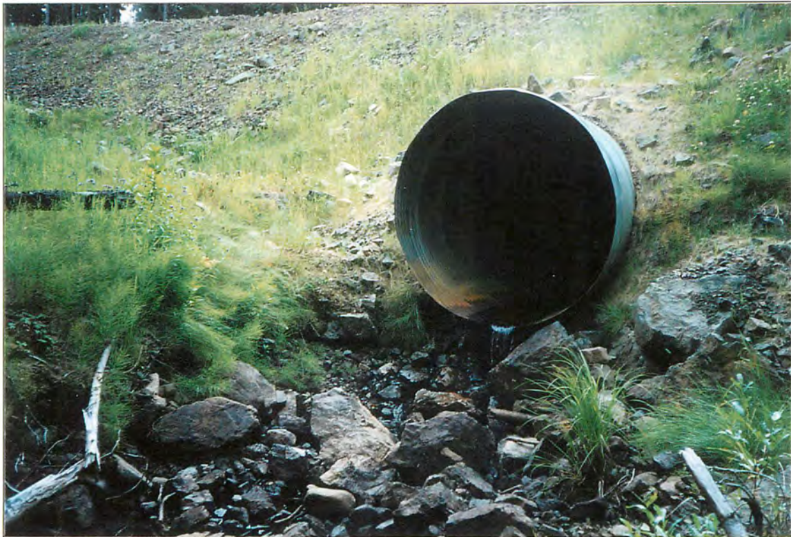
Site #21, Photo of perched culvert. Roll #2, Frame #22A, Date: 2002/08/28
