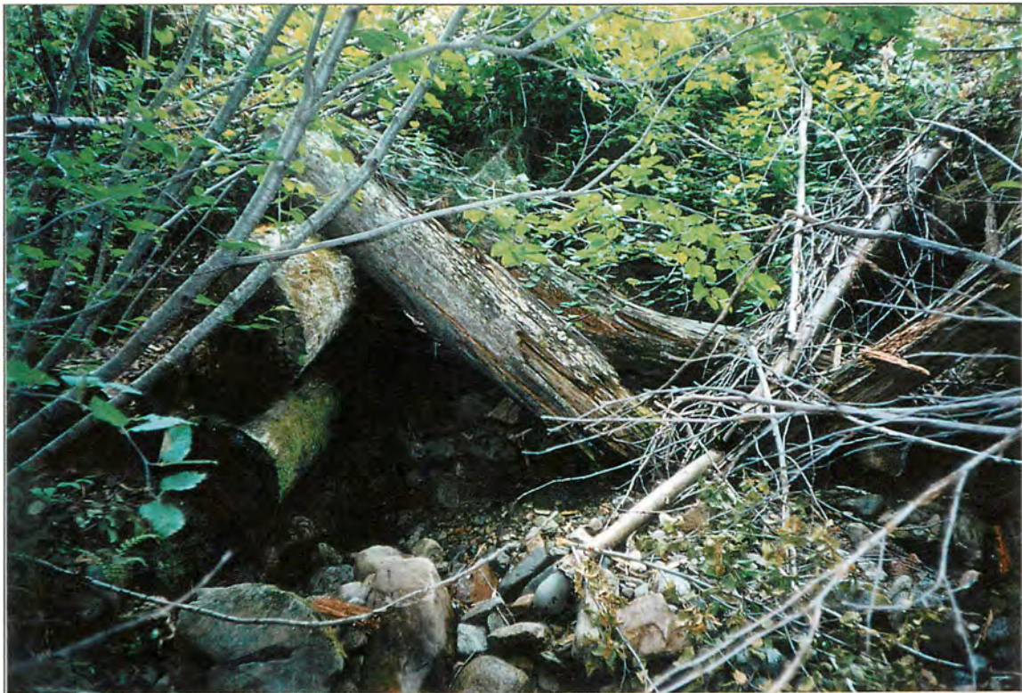
Site #15, Partially collapsed wooden culvert. Roll #2, Frame #6A, Date: 2002/08/28
