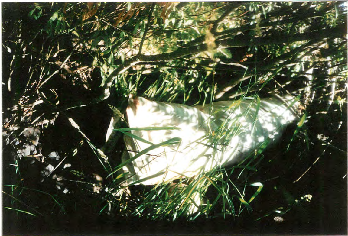
Site #988, Private culvert (damaged) 450 mm at 12% slope. Roll #93, Frame #18, Date: 2002/09/09
