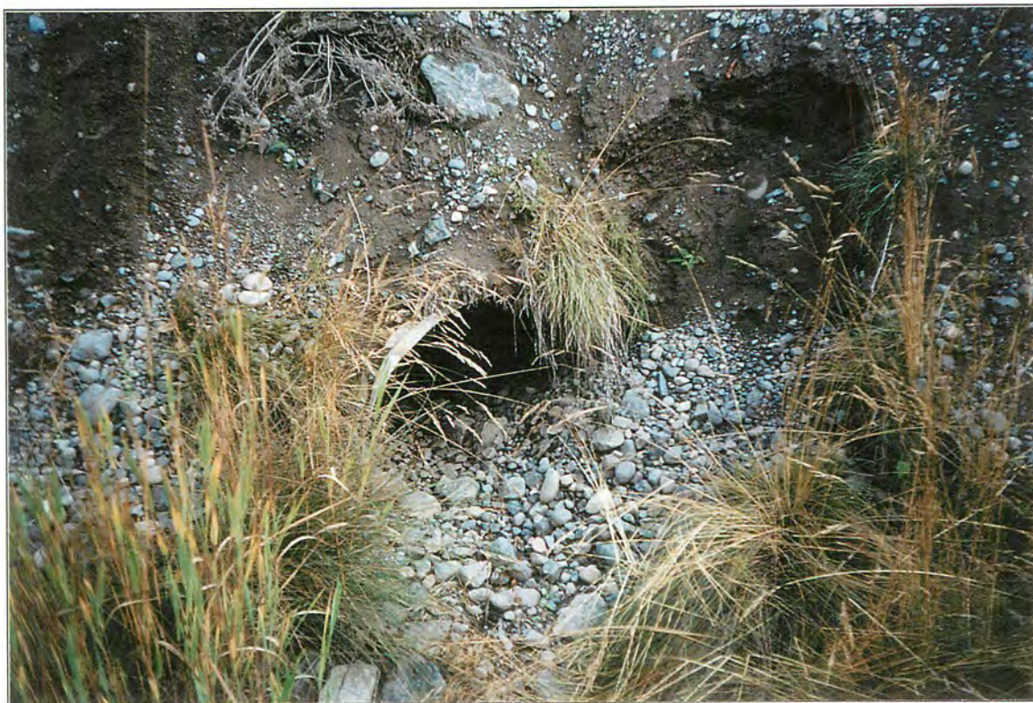
Site #918, Culvert at road slight bank failure. Roll #52, Frame #04, Date: 2002/09/05
