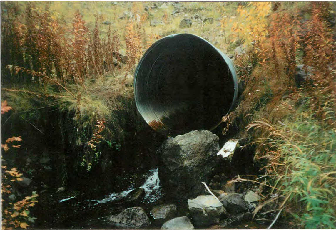
Site #624, Culvert at road crossing perched 1 m (high priority). Roll #63, Frame #17, Date: 2002/09/27
