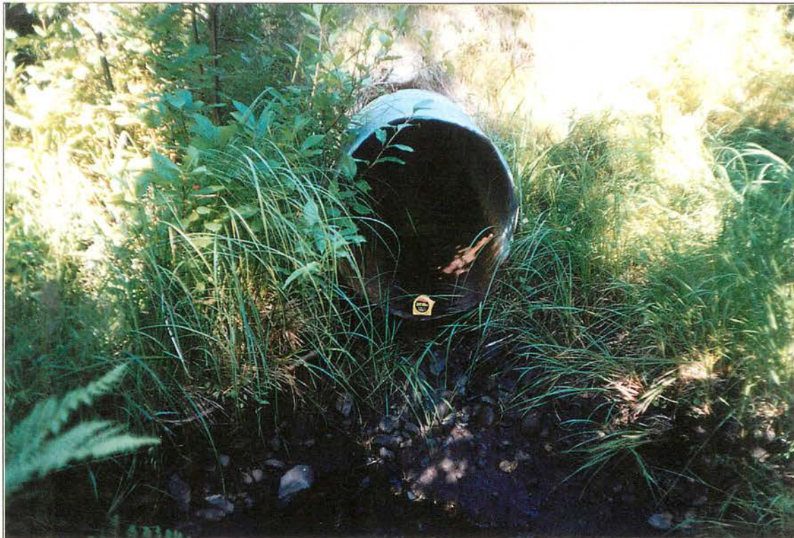
Site #533, Culvert at road crossing perched 40 cm. Roll #54, Frame #08, Date: 2002/09/06
