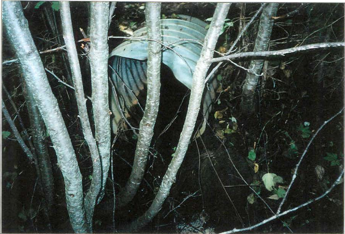
Site #558, Culvert outlet perched and blocked. Roll #57, Frame #12, Date: 2002/09/10
