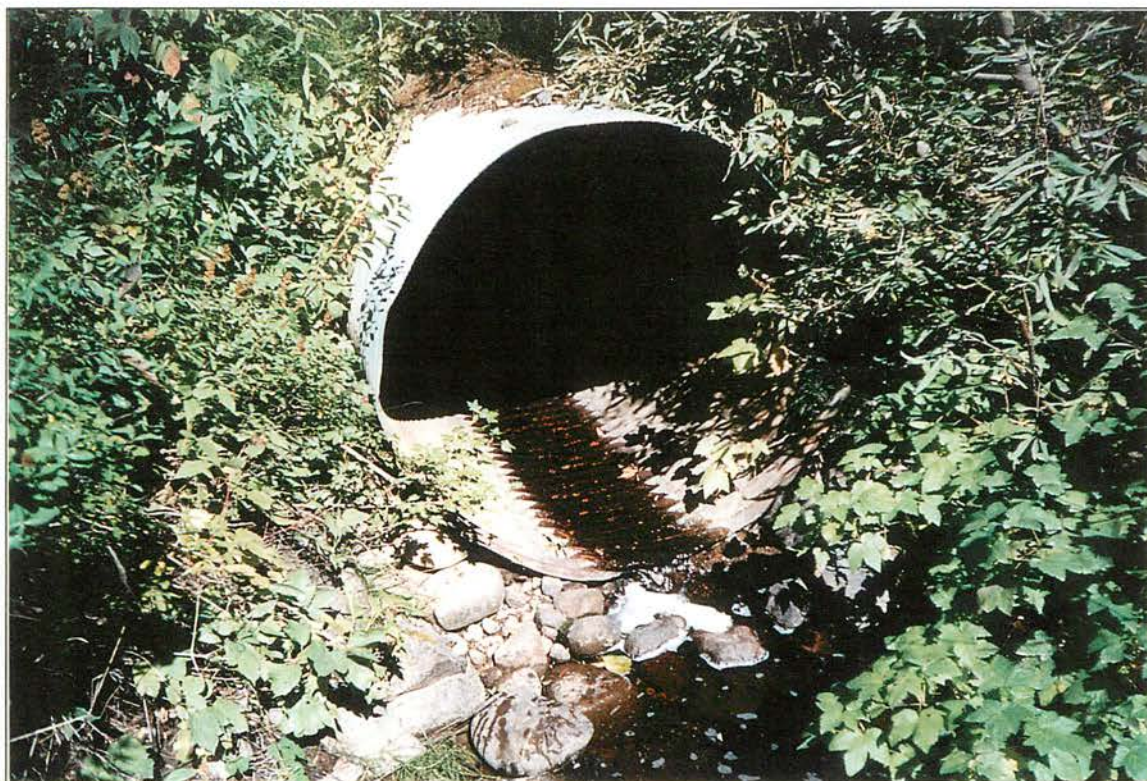
Site #532, Culvert outlet, perched 10 cm. Roll #54, Frame #07, Date: 2002/09/06
