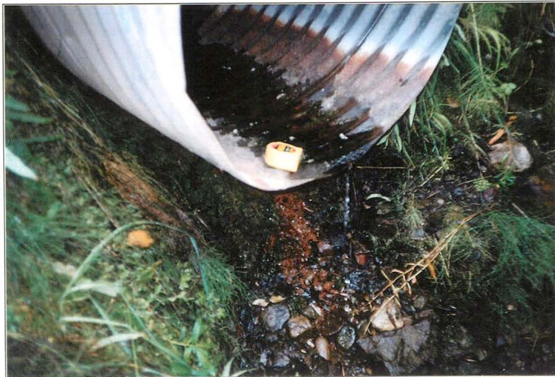
Site #503, Culvert perched 1 m. Roll #50, Frame #13, Date: 2002/09/03
