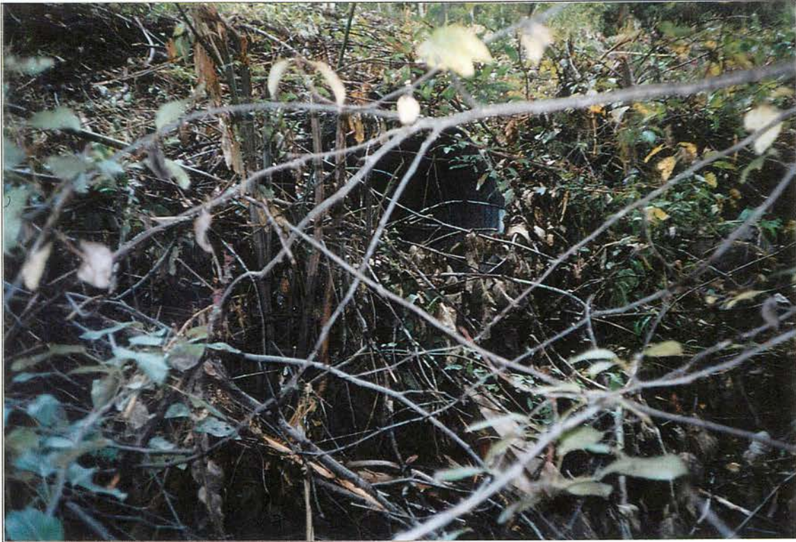
Site #501, Culvert outlet perched 1 m. Roll #50, Frame #05, Date: 2002/09/03
