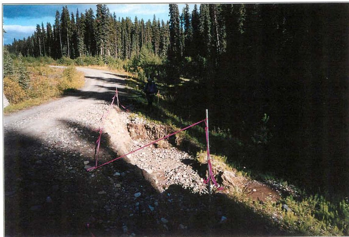
Site #527, Road erosion. Roll #53, Frame #09, Date: 2002/09/05
