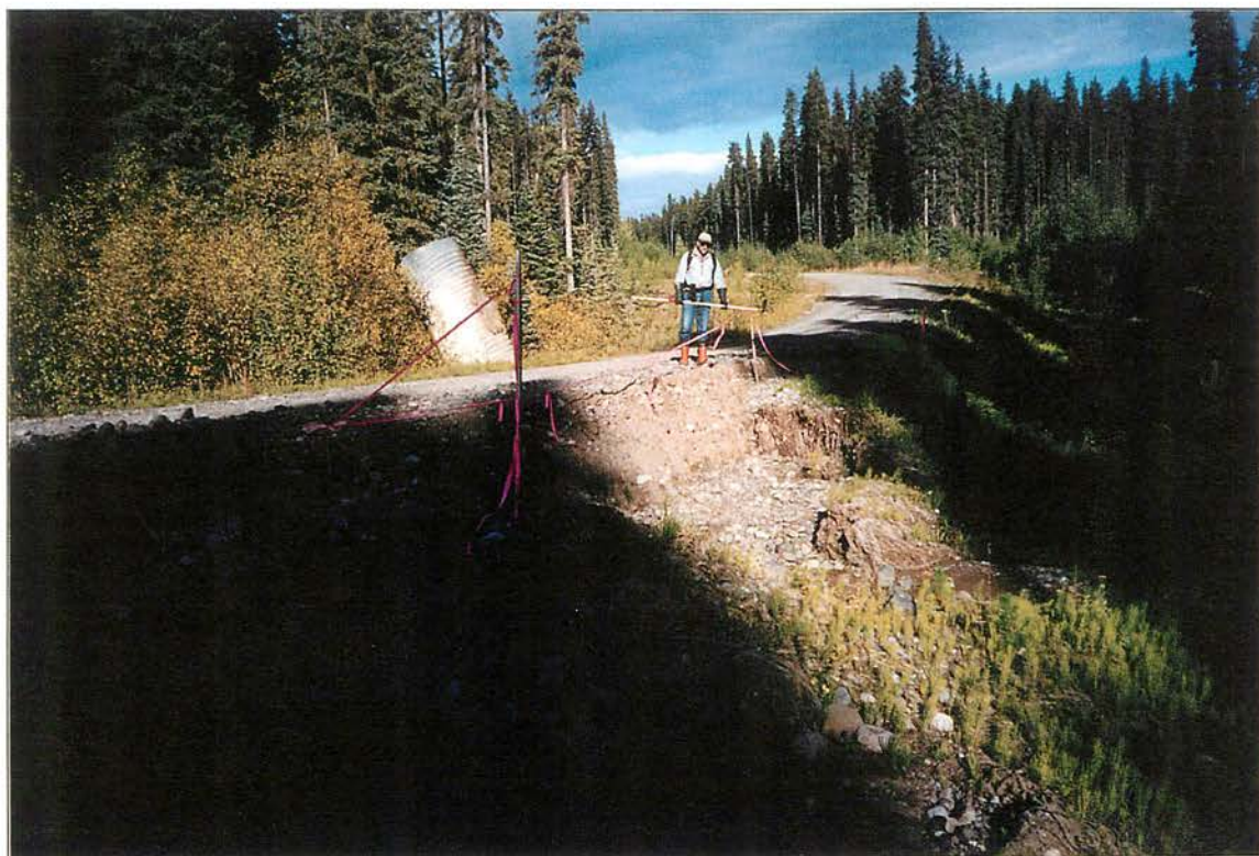
Site #527, Road erosion. Roll #53, Frame #08, Date: 2002/09/05
