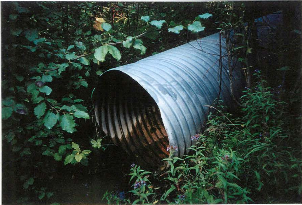
Site #521, Culvert perched 50 cm. Roll #52, Frame #13, Date: 2002/09/05
