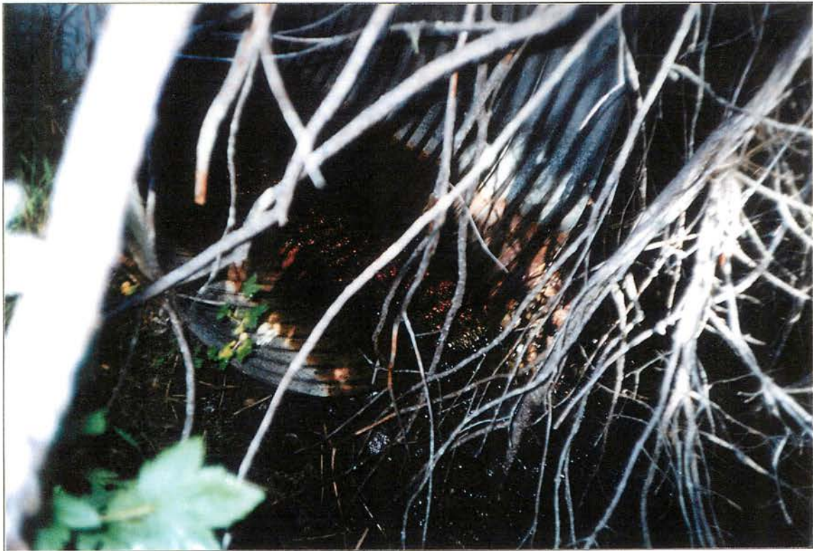
Site #520, Perched culvert (30 cm) higher than average gradient ~6% (estimated visual observation). Roll #52, Frame #08, Date: 2002/09/05
