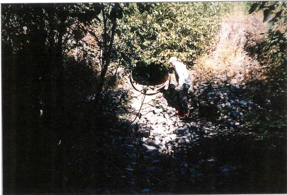
Site #519, Upstream photo at culvert outlet perched / expanded / slump / high velocity. Roll #52, Frame #07, Date: 2002/09/05
