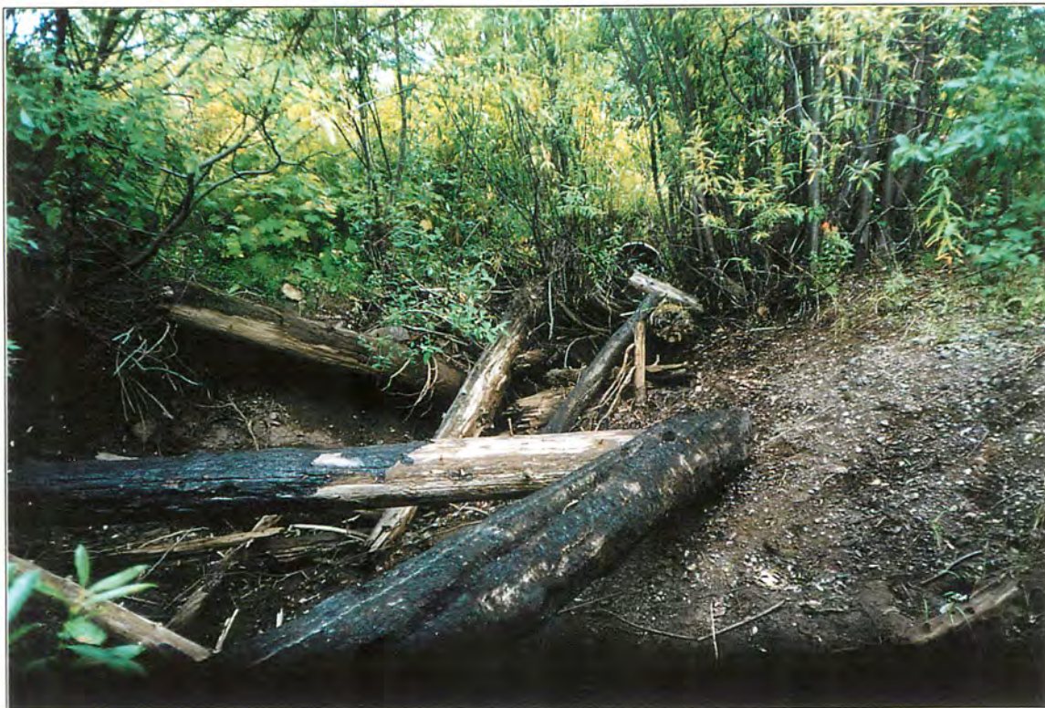
Site #276, Downstream photo of culvert inlet (disturbed section) ponded area due to perched inlet. Roll #96, Frame #05A, Date: 2002/09/05
