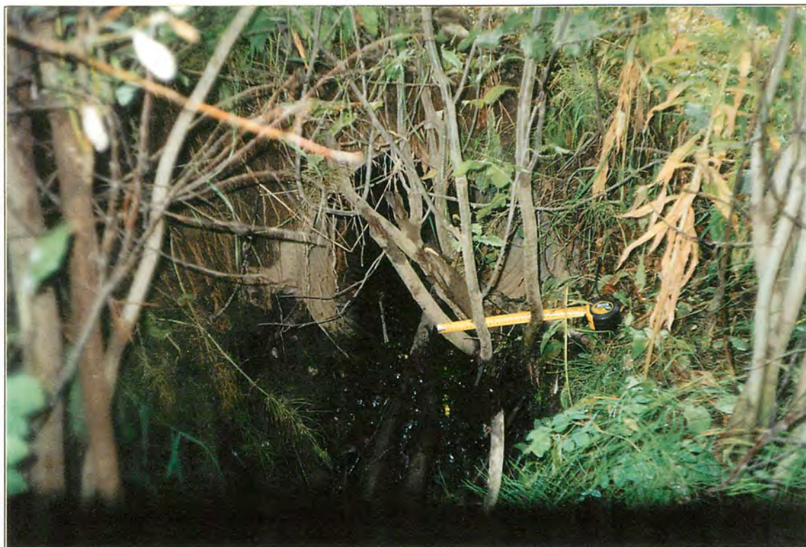
Site #252, Upstream photo of 0.2 m perched culvert (partial barrier). Roll #99, Frame #09, Date: 2002/09/03
