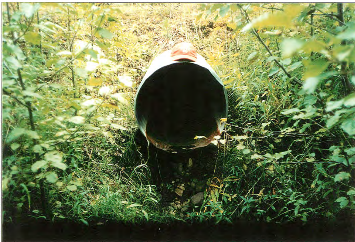
Site #284, Upstream photo of 0.8 m perched culvert. Roll #95, Frame #04, Date: 2002/09/06
