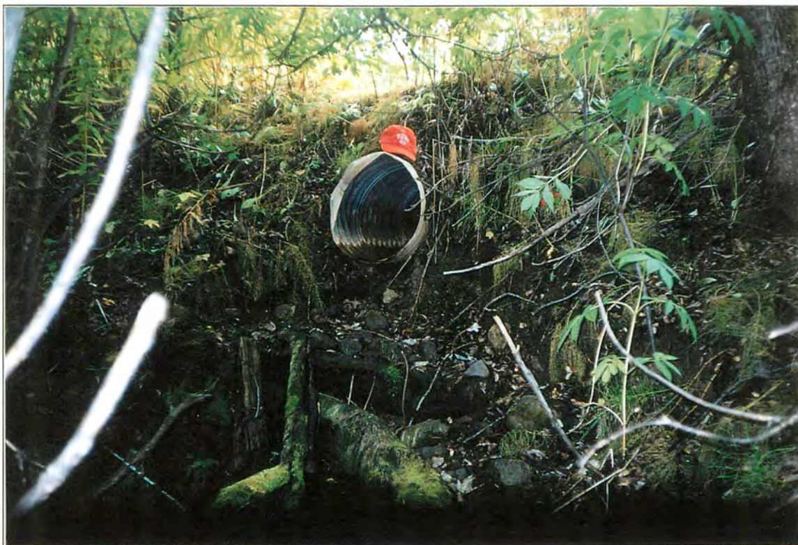
Site #276, Upstream photo of culvert perched ~2.0 m. Roll #96, Frame #02A, Date: 2002/09/05
