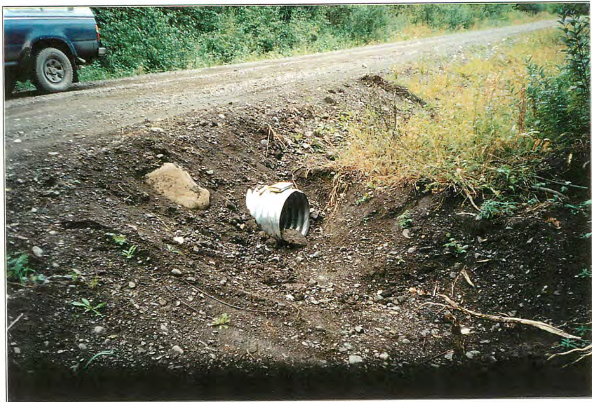
Site #256, Upstream photo of 0.4 x 12 m culvert (with book). Roll #99, Frame #19, Date: 2002/09/03
