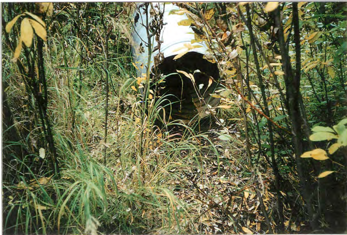
Site #82, Downslope photo of seepage. Roll #7, Frame #14A, Date: 2002/09/27
