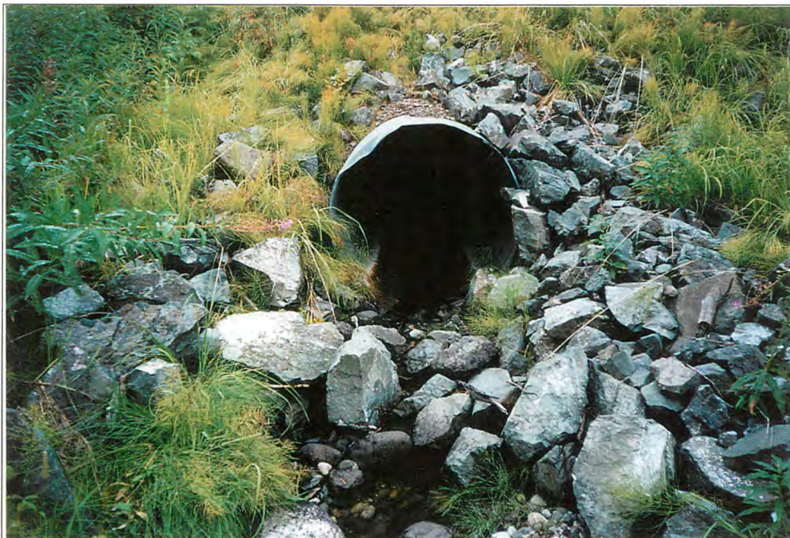
Site #48, Photo of culvert - gradient too high. Roll #6, Frame #01A, Date: 2002/09/03
