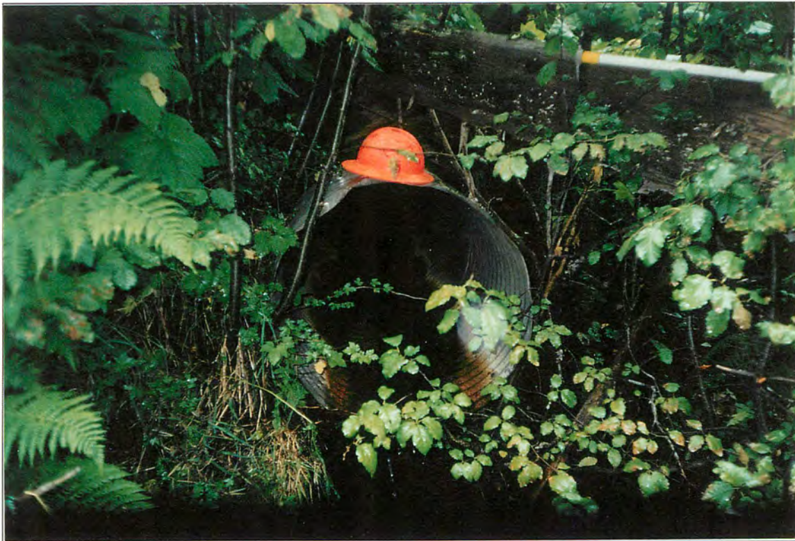
Site #268, Upstream photo of 0.5 m perched culvert. Roll #97, Frame #01, Date: 2002/09/04
