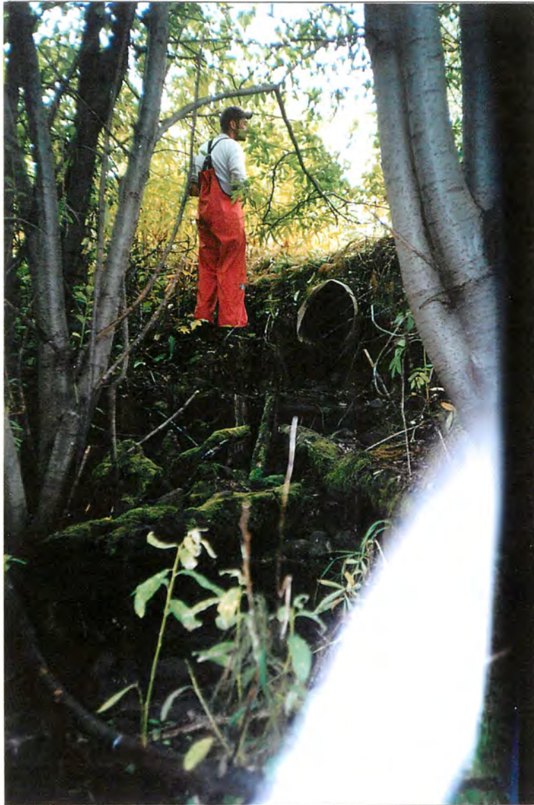
Site #276, Upstream photo of culvert outlet perched ~2.0 m. Roll #96, Frame #06A, Date: 2002/09/05
