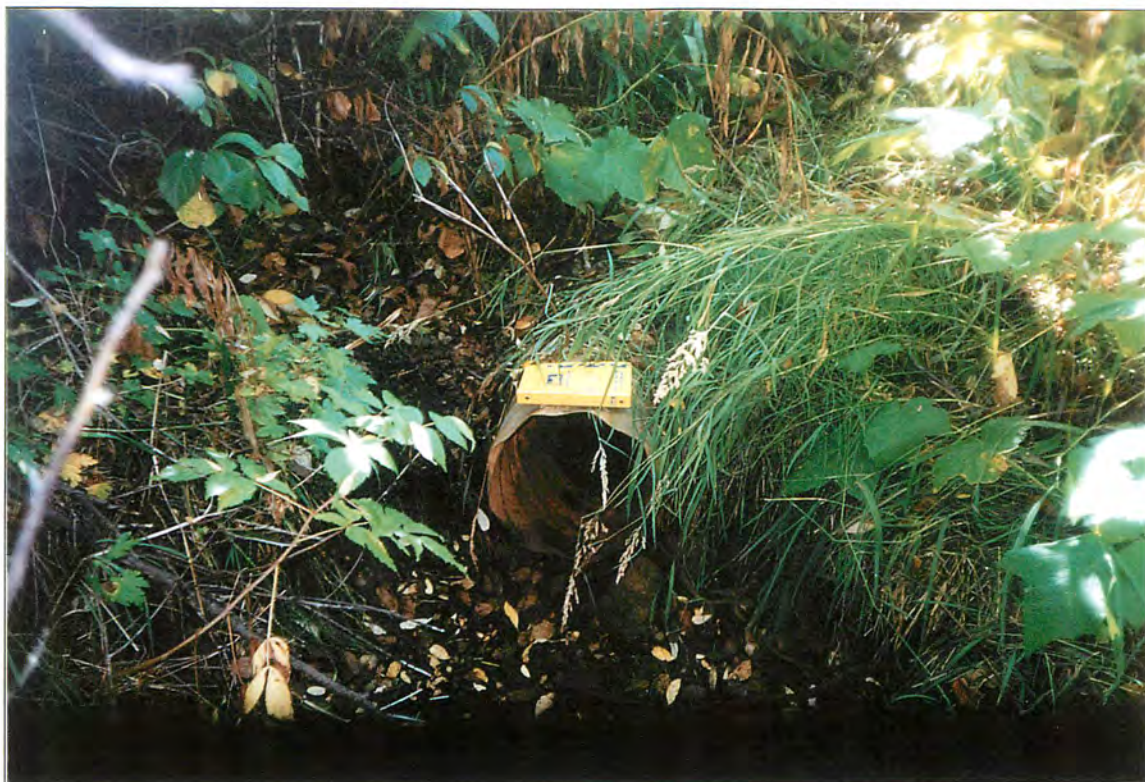
Site #277, Upstream photo of 0.20 m perched culvert. Roll #96, Frame #07A, Date: 2002/09/05
