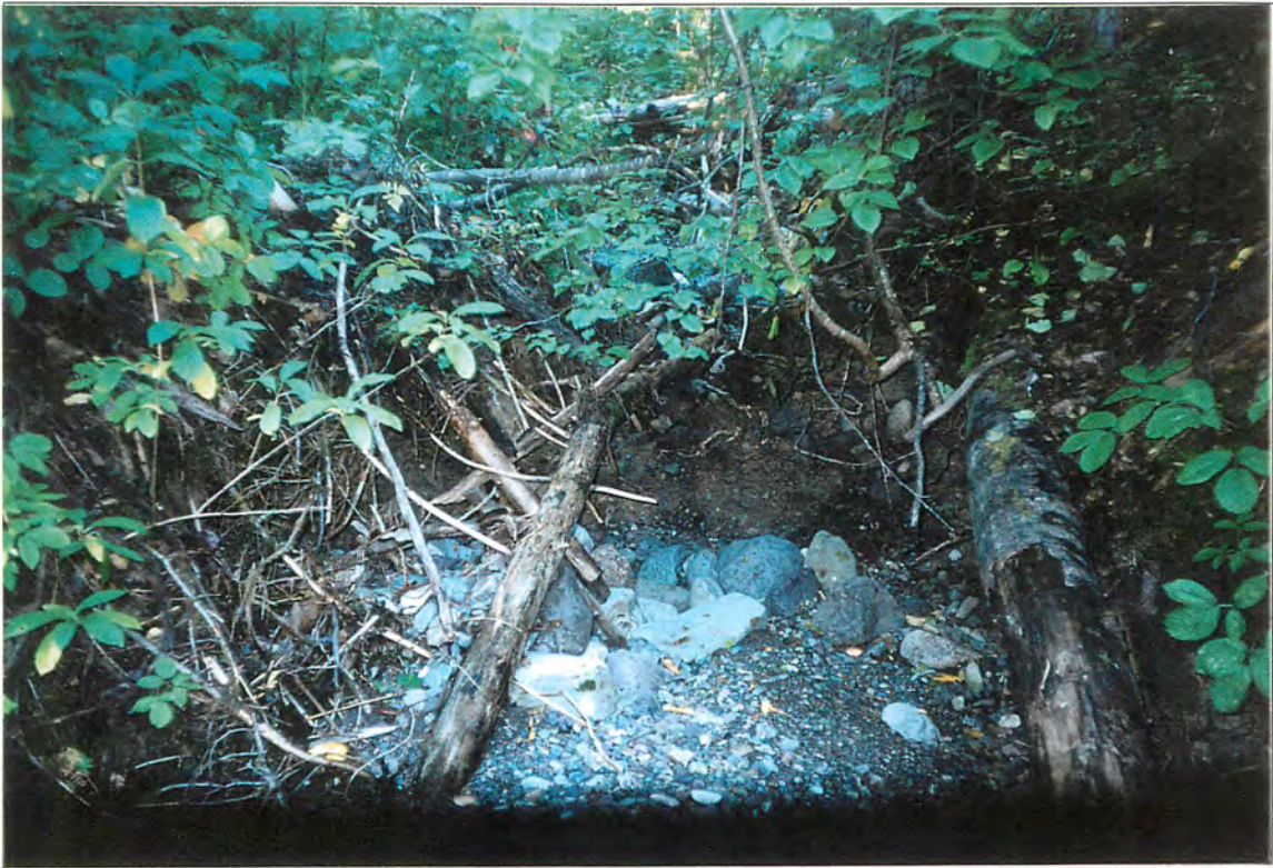
Site #279, Upstream photo showing non-permanent obstruction. Roll #96, Frame #13A, Date: 2002/09/06
