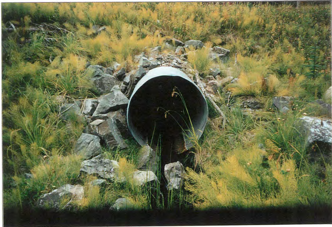
Site #308, Upstream photo of perched 0.10 m culvert. Roll #92, Frame #12, Date: 2002/09/11
