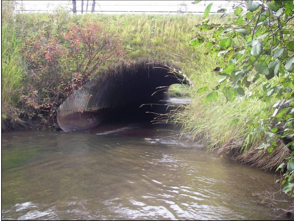
Figure 5. View downstream to inlet, inlet is flush with stream bed (September 24, 2011).
