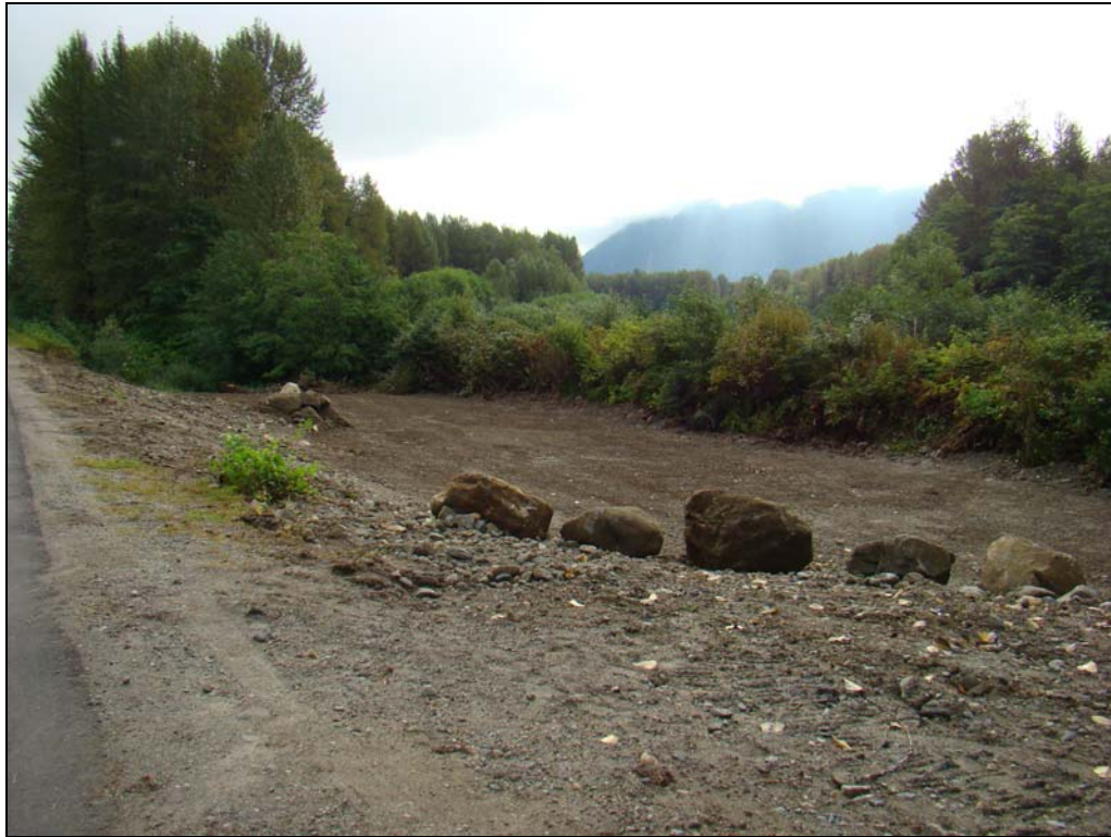
Figure 11 – Backfilling completed at the area between the highway and railway at Site 4.
