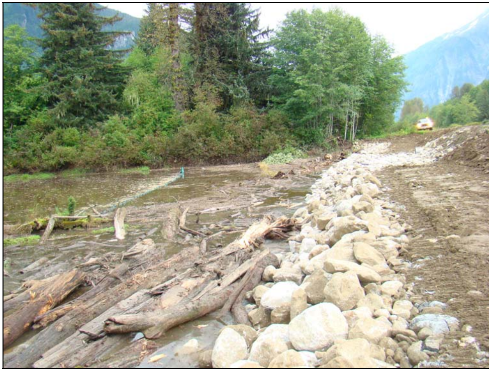
Figure 12 – The grade seal being constructed on the north side of Site 2 where there is a 600 mm culvert through the road & rail grade.
