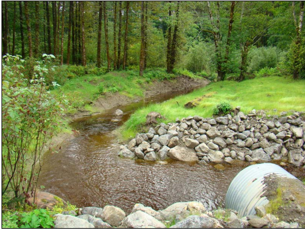
Figure 15 – A view of the outlet area downstream of the culverts put in at Site 3 by CN. A low weir has been added to the outlet channel. Note the vegetation cover has been restored by hydroseeding.
