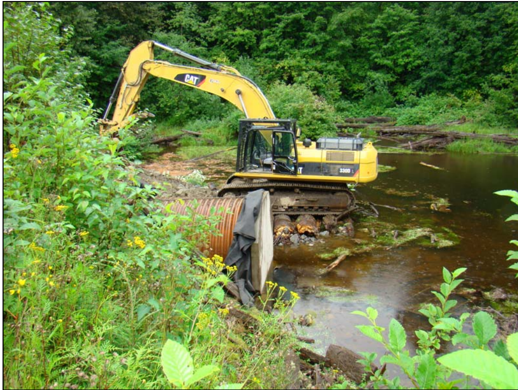
Figure 9: Sealing off the culvert at Site 4 (Death Hole) on the north side of the highway. The photo shows the concrete cap in place before the area was sealed off with backfill.
