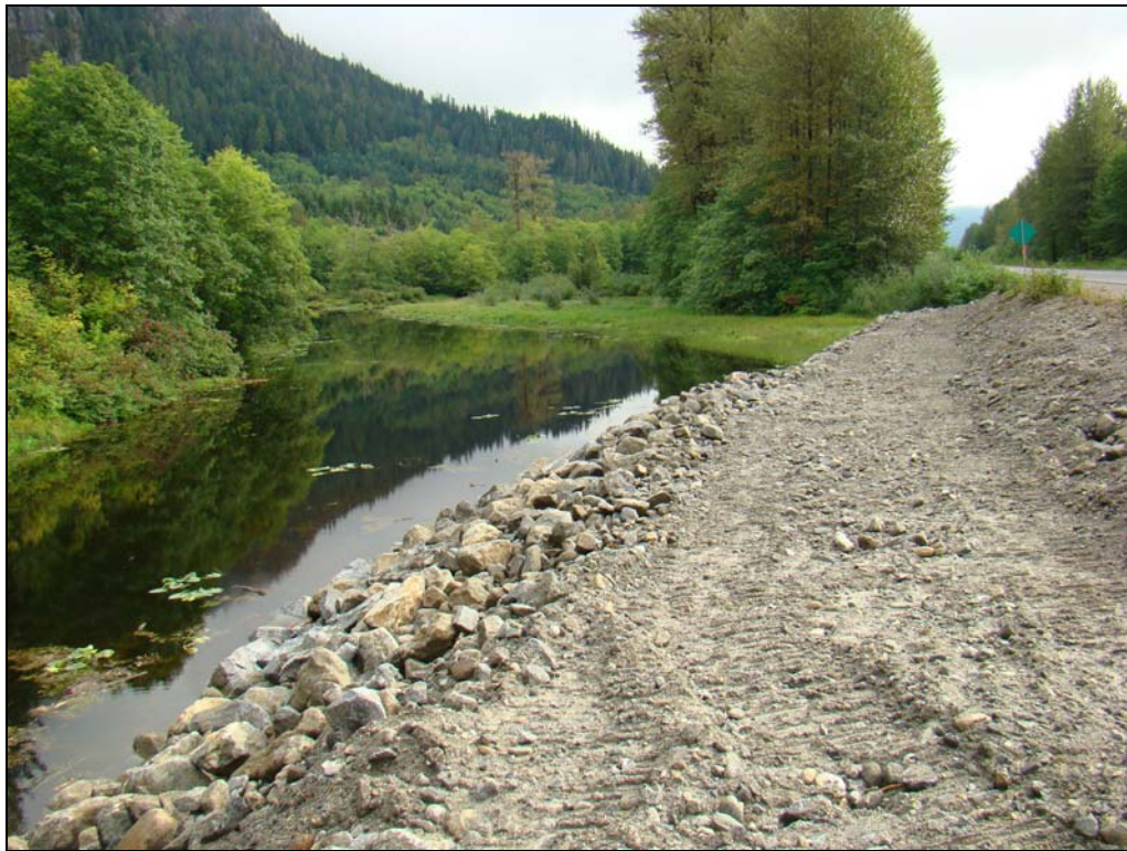
Figure 10: The completed grade seal at the north end of the highway culvert at Site 4.
