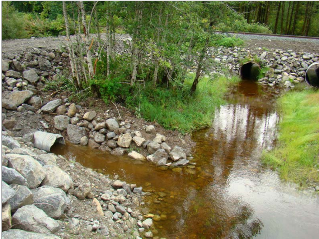
Figure 14 – An additional culvert was inserted into the east CN berm at Site 3.
