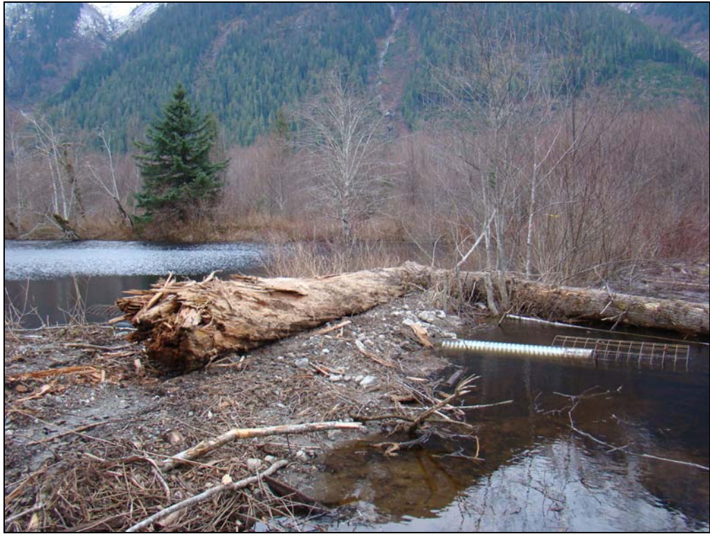
Figure 16 – Beaver stops on both ends of a culvert installed through an old corduroy bridge. This location was identified in the original studies as a partial barrier to fish movement within the project. The beaver stops alleviate this problem.
