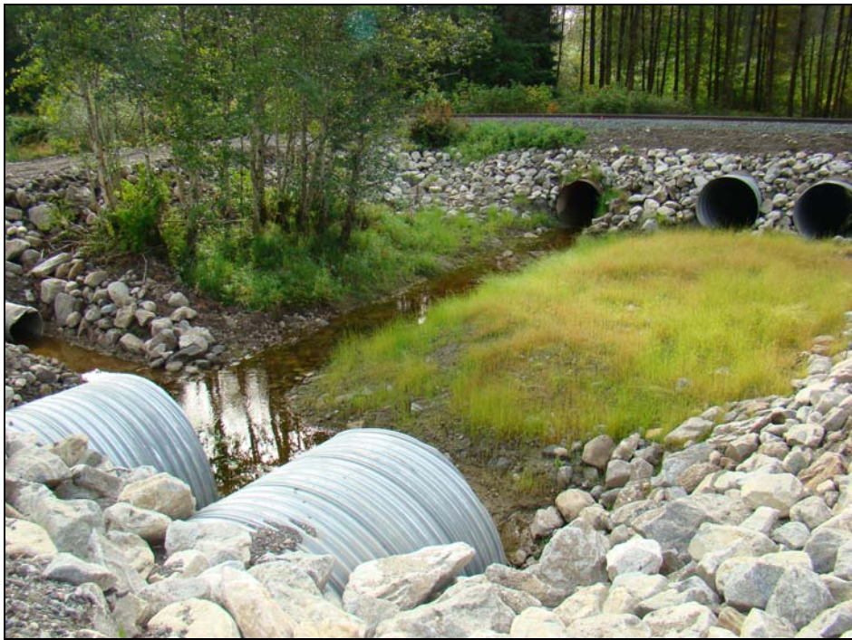
Figure 5: Site 3, looking downstream at the section between the CN and MOT right of ways at the newly constructed sidechannel outlet. Work was done with the funding acquired in 2007 from MoT and CN. Photo taken in August 2008.
