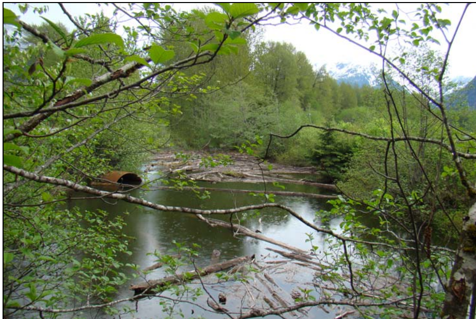
Figure 6: Site 4 (the Death Hole) on May 21, 2008. The visible (2600 mm diameter) culvert through the highway grade does not have a match through the railway grade (on the photo right). The isolated pool frequently stranded fish when the floodplain water levels dropped and the fish were unable to retreat back into the sidechannel due to the elevation of the culvert outlet.
