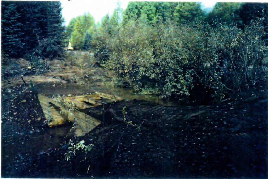
Photo 4. Laminated treated timber enumeration sill at outlet of pond complex. Culvert through road is in center of photo.
