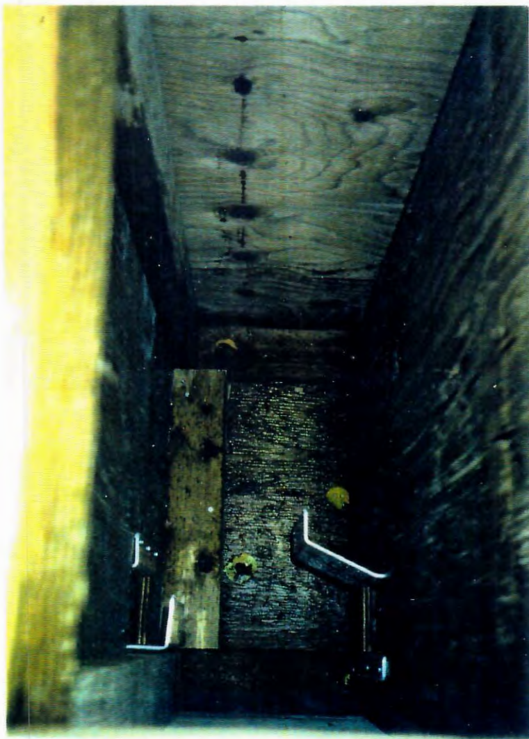
Photo 6. Inside view of baffle/port detail of fry fishway. Aluminum deflectors are screwed into plywood baffle at port. The port is 3.75 in x 8 in. high.
