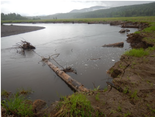
Photo 9. Bulkeley River at McKilligan Rd (Lower) – Upstream view of the damaged LWD structure (0+000 m) and groin (0+018 m; 19 July 2017).
