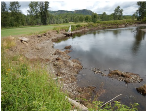
Photo 5. Bulkley River at Craker Rd (Lower) – Looking upstream from 0+015 m prior to construction (23 July 2017).
