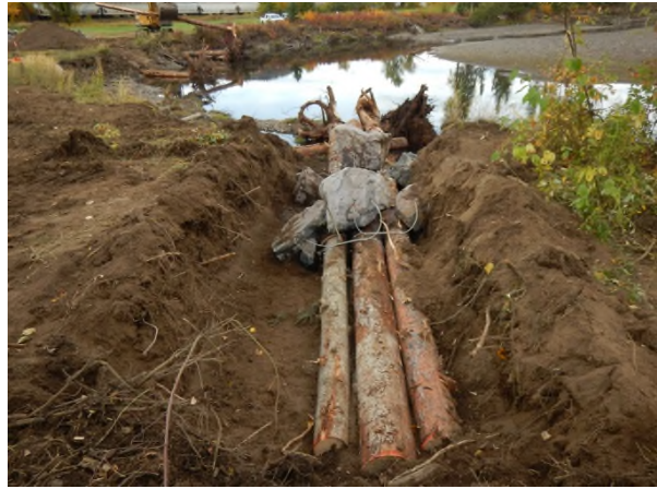
Photo 2. Bulkley River at Craker Rd (Lower) – Ballasted logs in the upstream-facing trench of the LWD structure at 0+030 m (26 September 2017).
