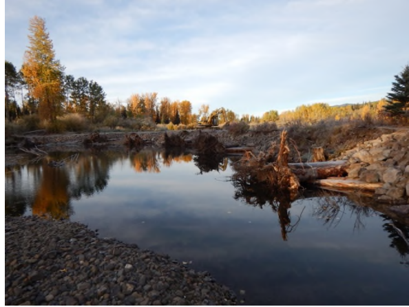
Photo 8. Bulkeley River at Craker Rd (Lower) – Looking downstream from 0+090 m after construction was completed (3 October 2017).
