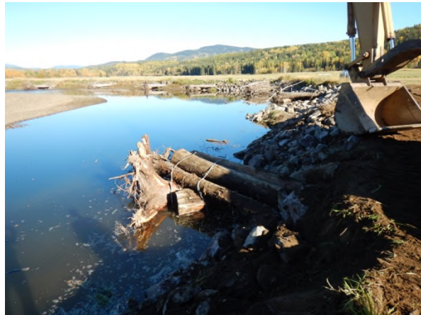
Photo 10. Bulkeley River at McKilligan Rd (Lower) – Upstream view of the repaired LWD structure (0+000 m) and groin (0+018 m; 2 October 2017).
