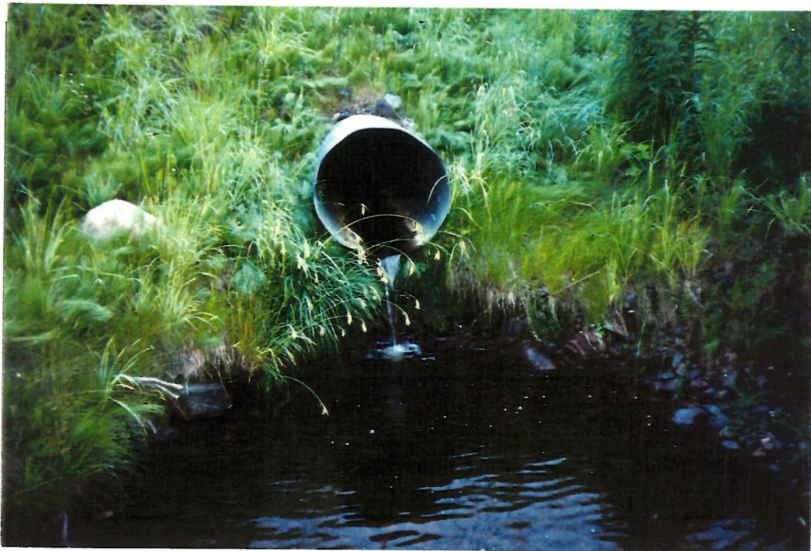
Photo #: 16 - 1 Site 167, upstream view of perched culvert at road crossing.
