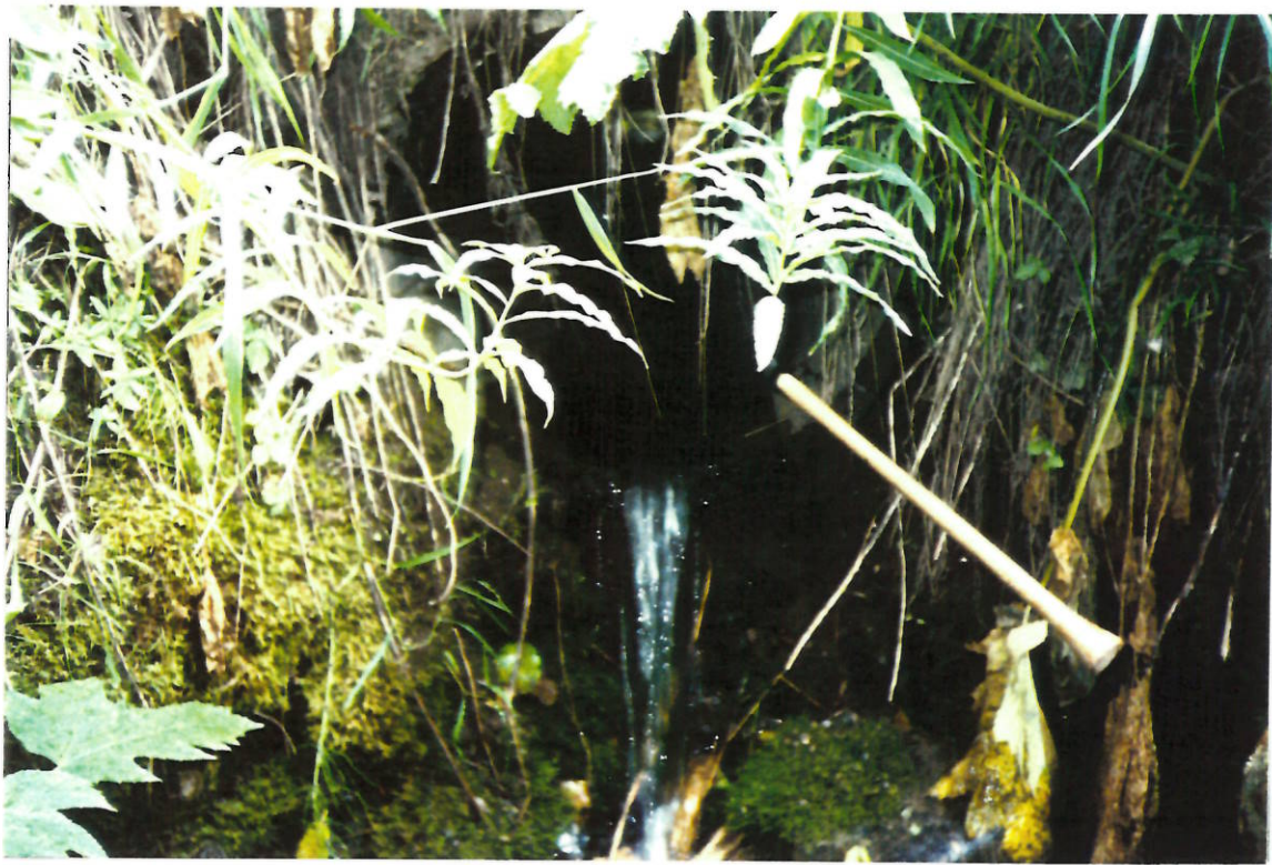
Photo #: 15 - 3 Site 157, view upstream of partial barrier at road crossing (0.8 m drop).
