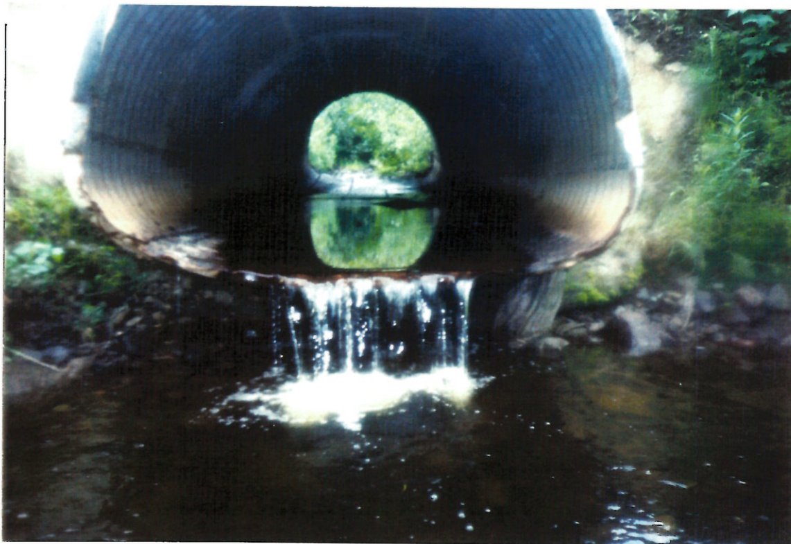
Photo #: 4 - 12 Site 341, looking upstream at culvert 2.9m with slight prop.
