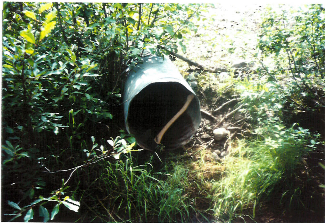
Photo #: 4 - 3 Site 339, looking upstream at culvert-slightly perched.
