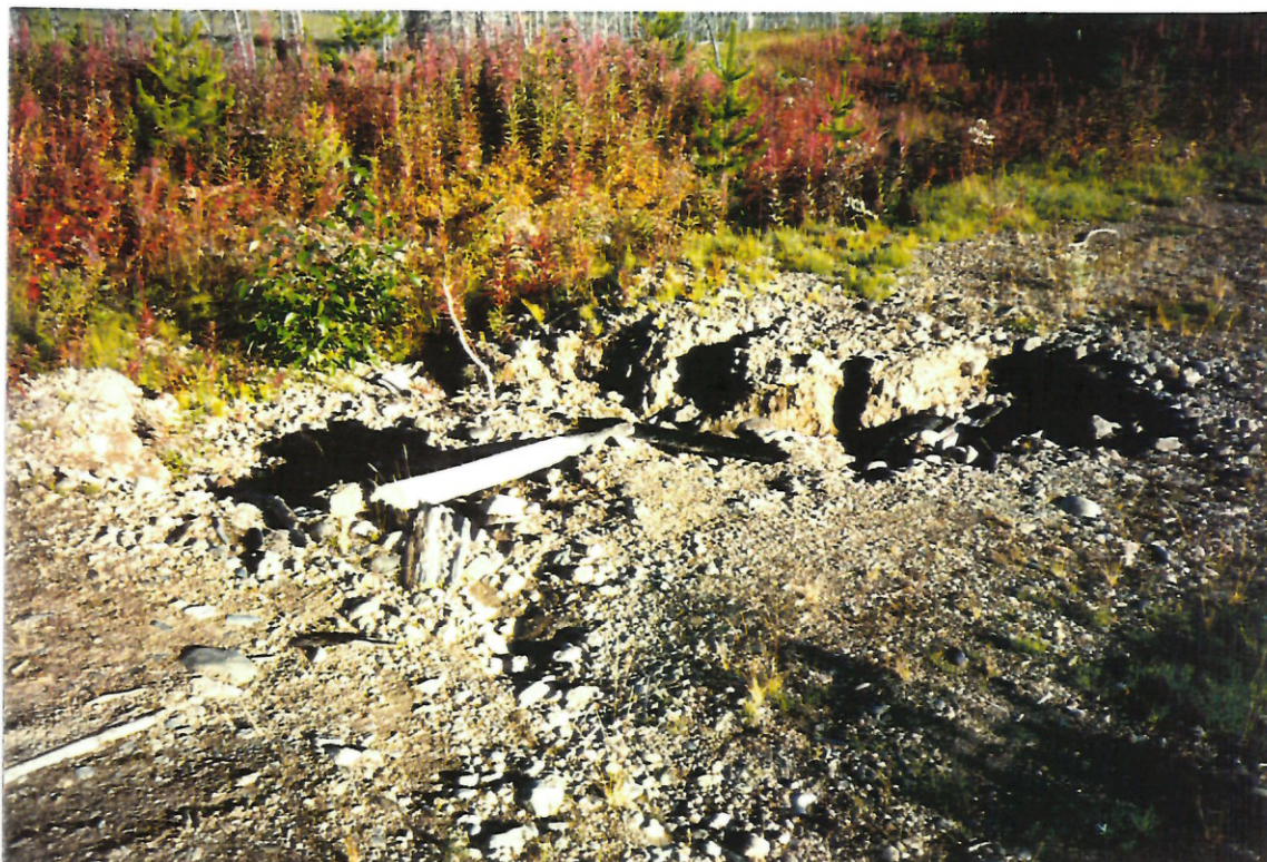
Photo #: 9 - 7 Site 392, erosion caused by blocked CV.
