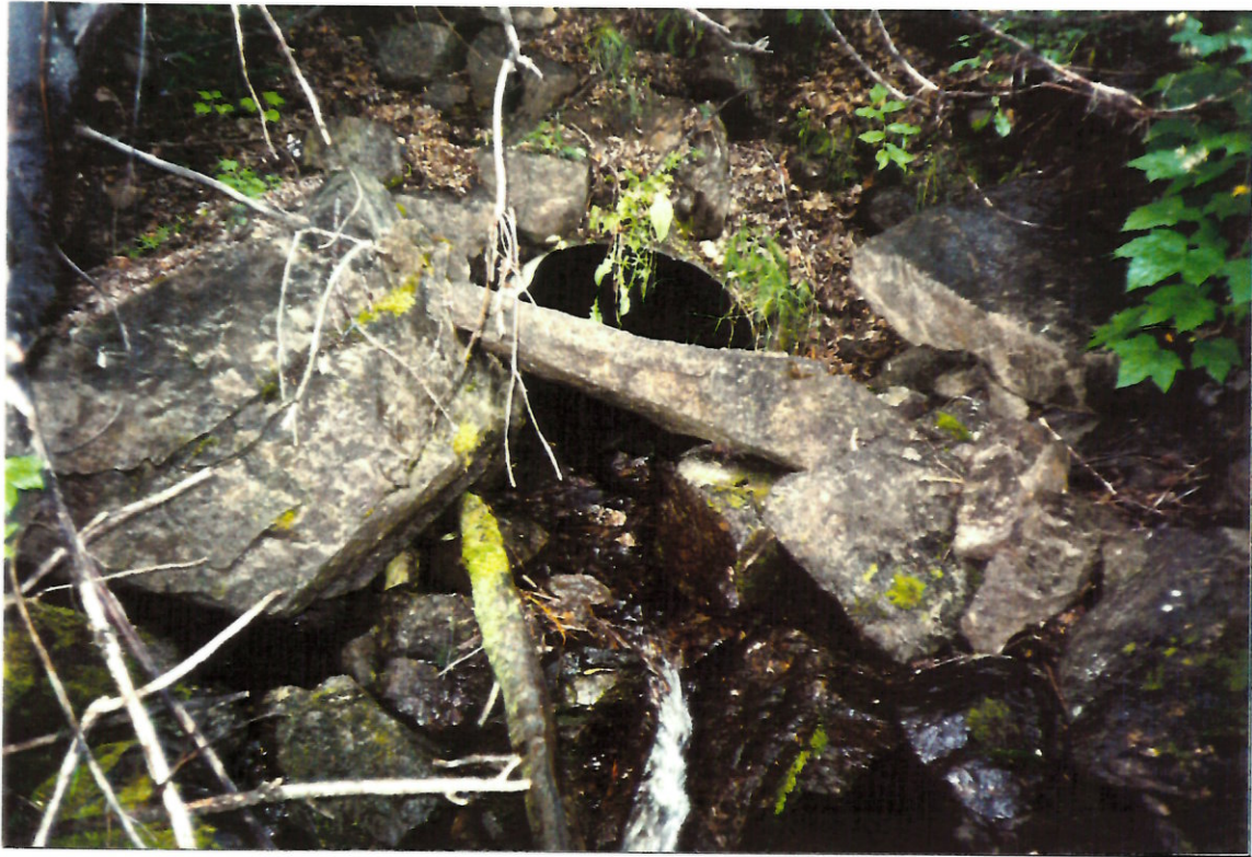
Photo #: 5 - 2 Site 351, looking upstream at 1m culvert - cascade at outlet partial barrier.
