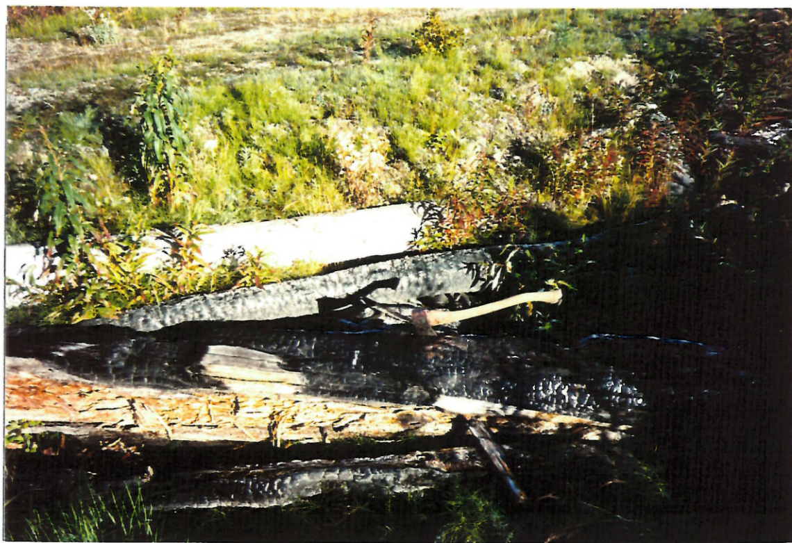
Photo #: 9 - 6 Site 392, looking downstream at CV blocked with woody debris, barrier to fish (axe).
