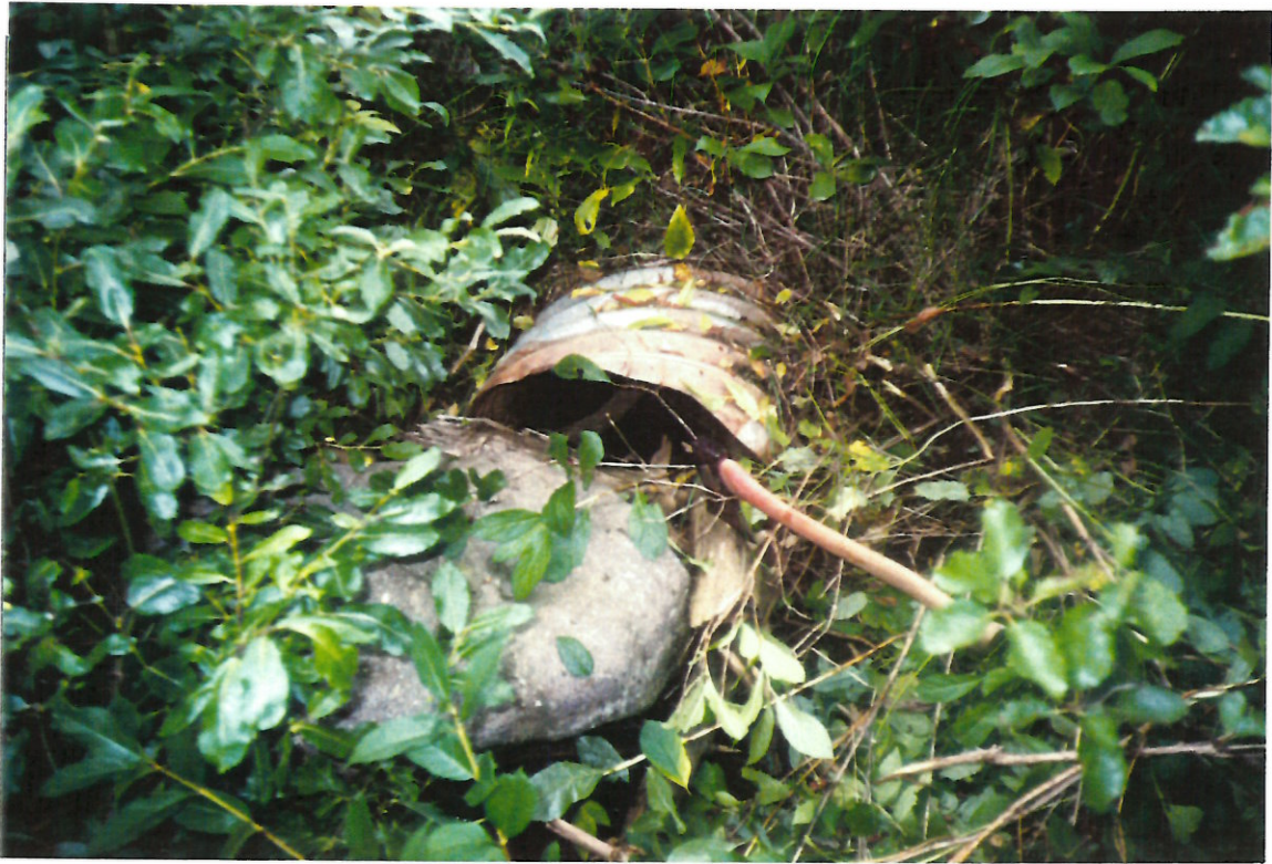
Photo #: 3 - 36 Site 338, culvert (600 mm) blocked with debris.
