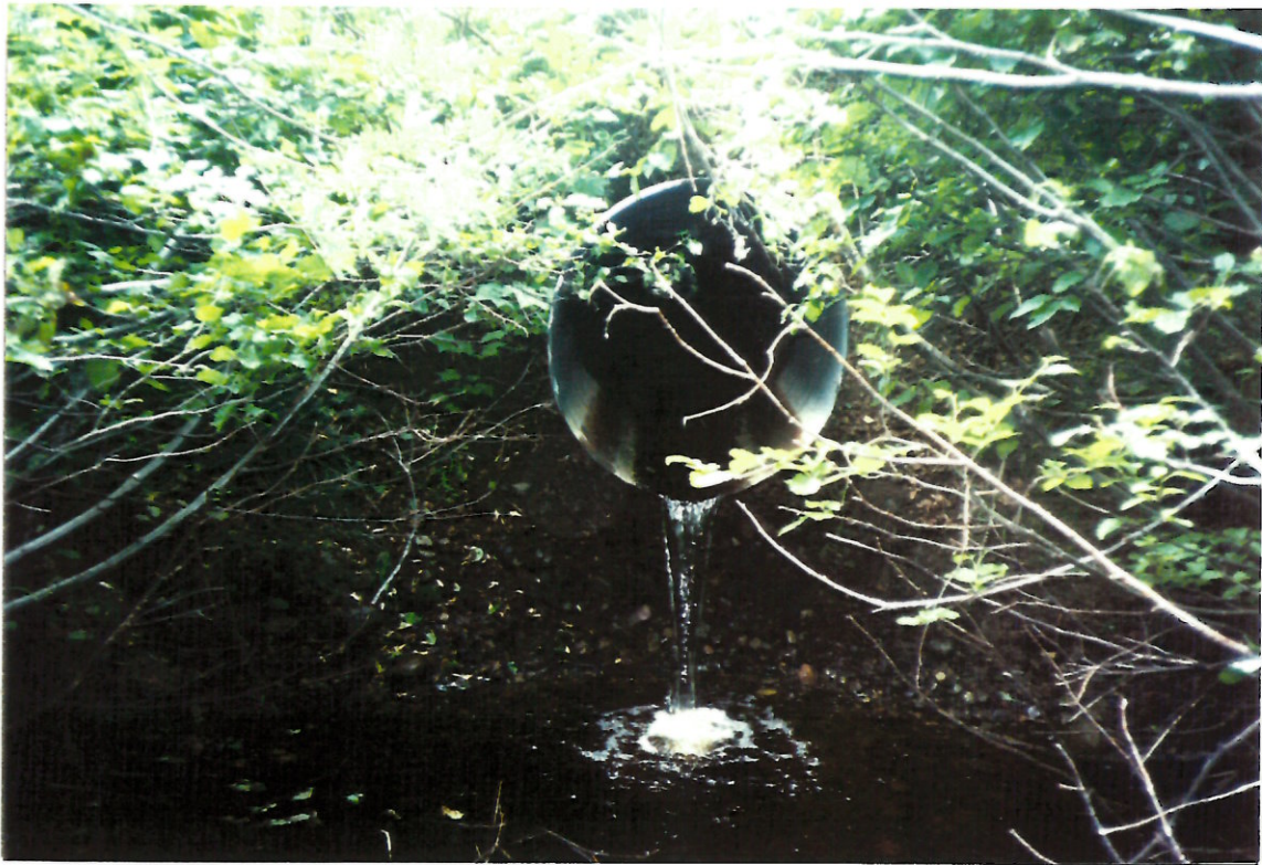
Photo #: 4 - 18 Site 344, looking upstream at culvert perched 80 cm, barrier during low flows.
