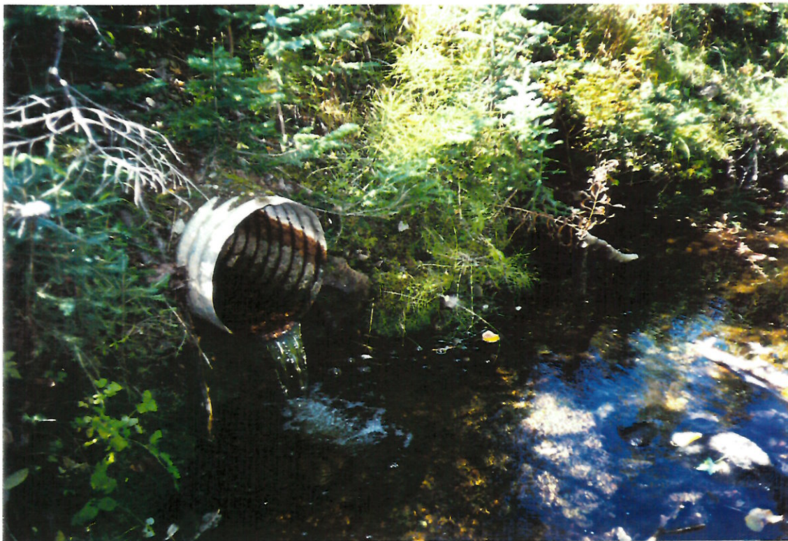
Photo #: 24 - 10 Site 253, upstream view of perched culvert (30 cm) with large pool downstream.
