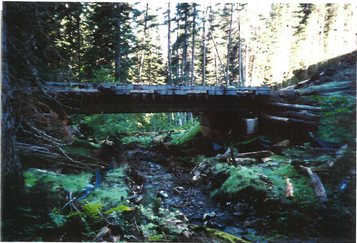
Photo #: 2 - 24 Site 318, looking downstream at bridge in poor shape - erosion.
