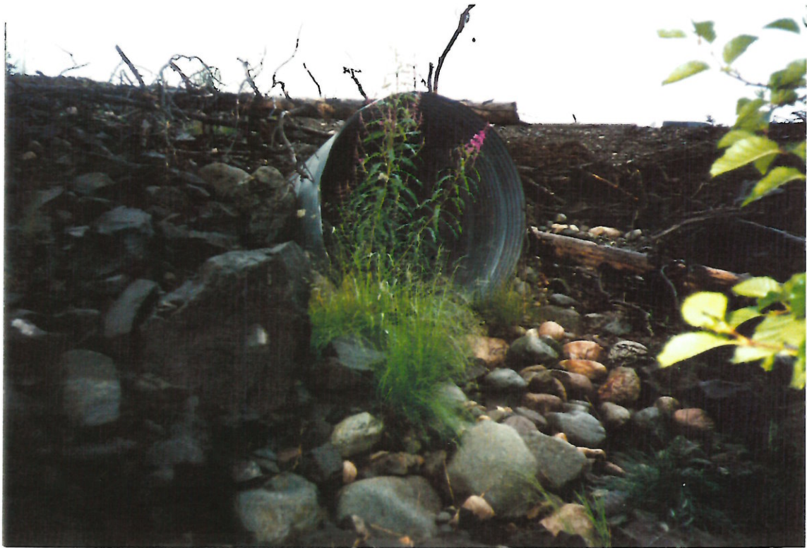
Photo #: 2 - 4 Site 311, looking upstream at culvert perched 2m CV (1.4m).
