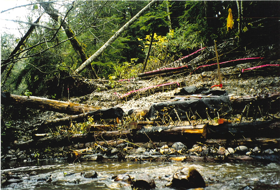
Photo 11: View from downstream of crib wall with live staking and bioengineering structures.
