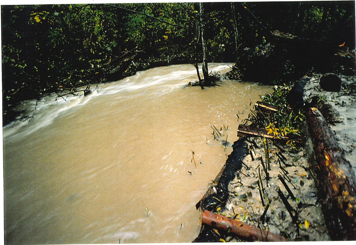
Photo 15: High water event in October showing crib wall structure protecting toe of slide.
