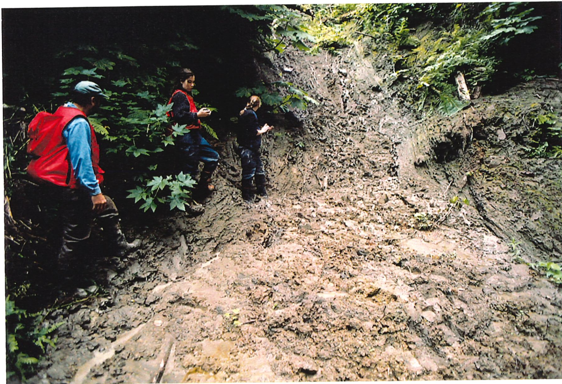
Photo 2: Lower end of transport zone, upper end of depositional zone prior to rehabilitation work.
