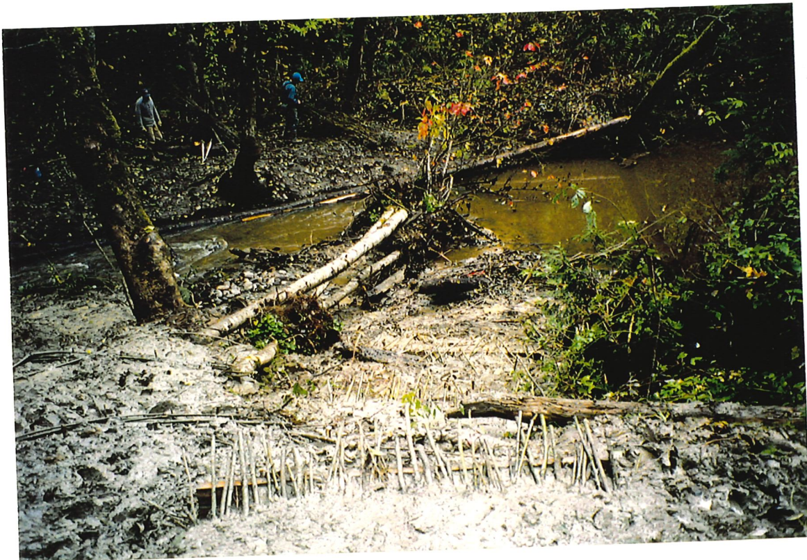
Photo 14: View of new channel showing LWD placements on right bank, modified brush layer (foreground).
